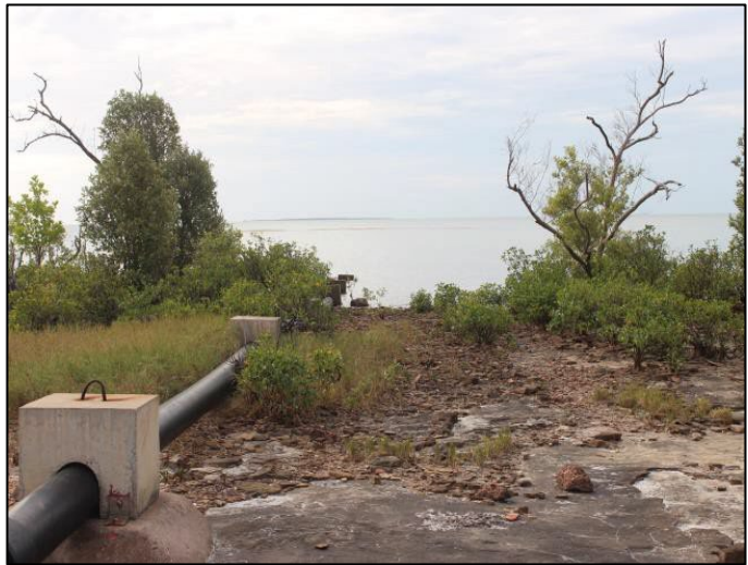
Figure 6: Maningrida Outfall (Power and Water 2016)
