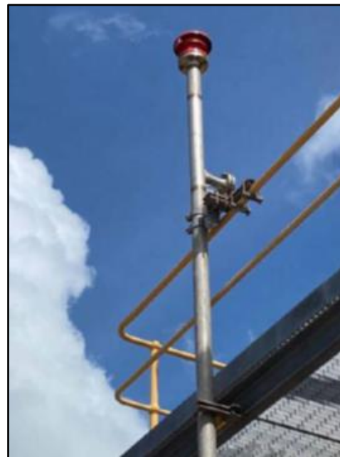
Figure 2: Scrubber Vent Stack
