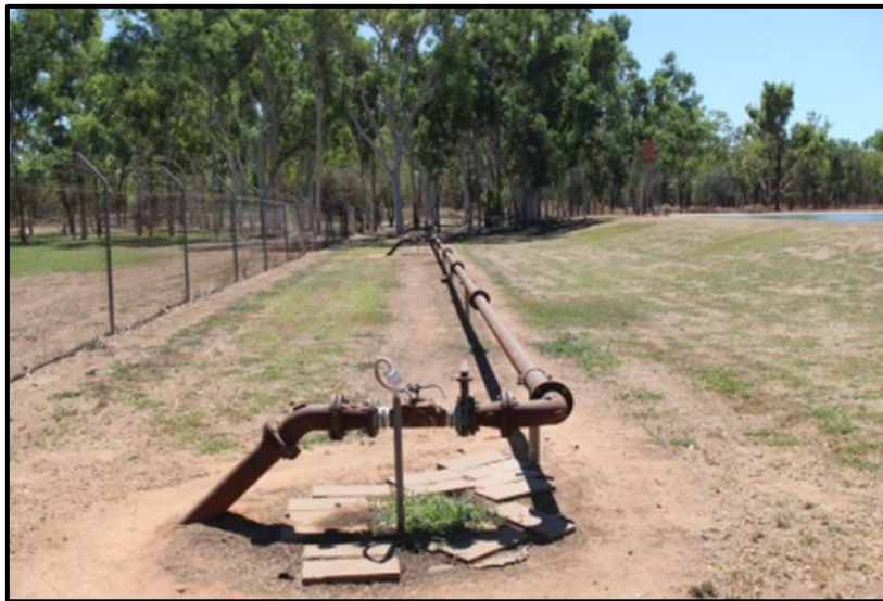
Figure 6. Beswick WwTP irrigation Pipeline (PWC 2017)
