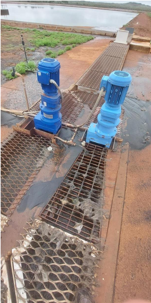
Appendix B – Location Photographs – macerators at inflow channel and where overflow occurred down embankment.
