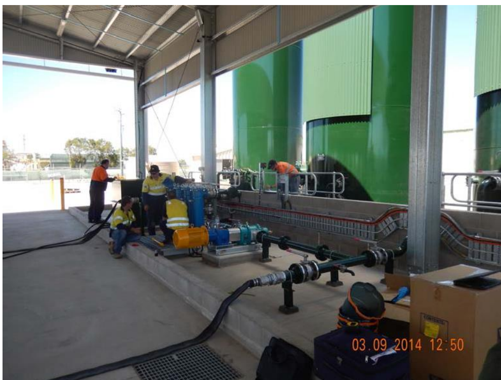
Plate 4 – Pump and Valve Bay
