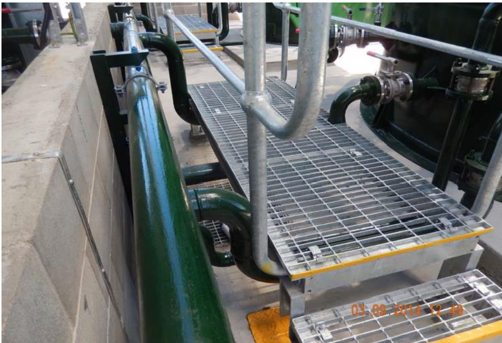
Plate 1 – Fixed Piping and Flanges
