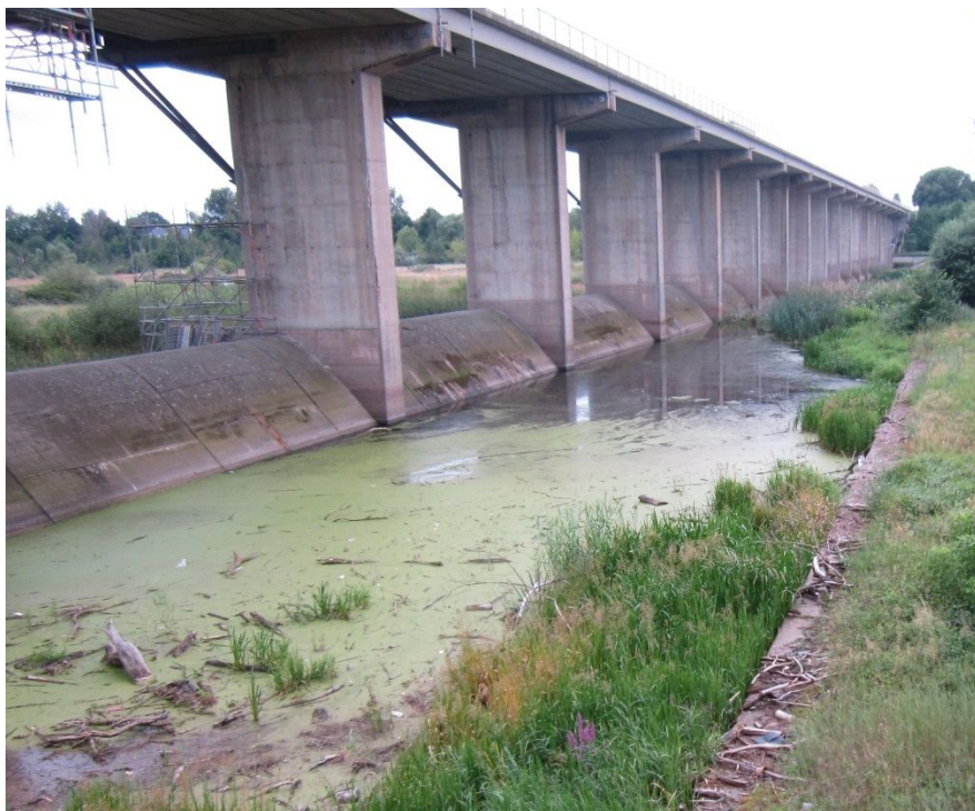
Figure 10. Flood inflow structure into Lake Zwenkau (Photo courtesy of Martin Schultze, Helmholtz Institute).
