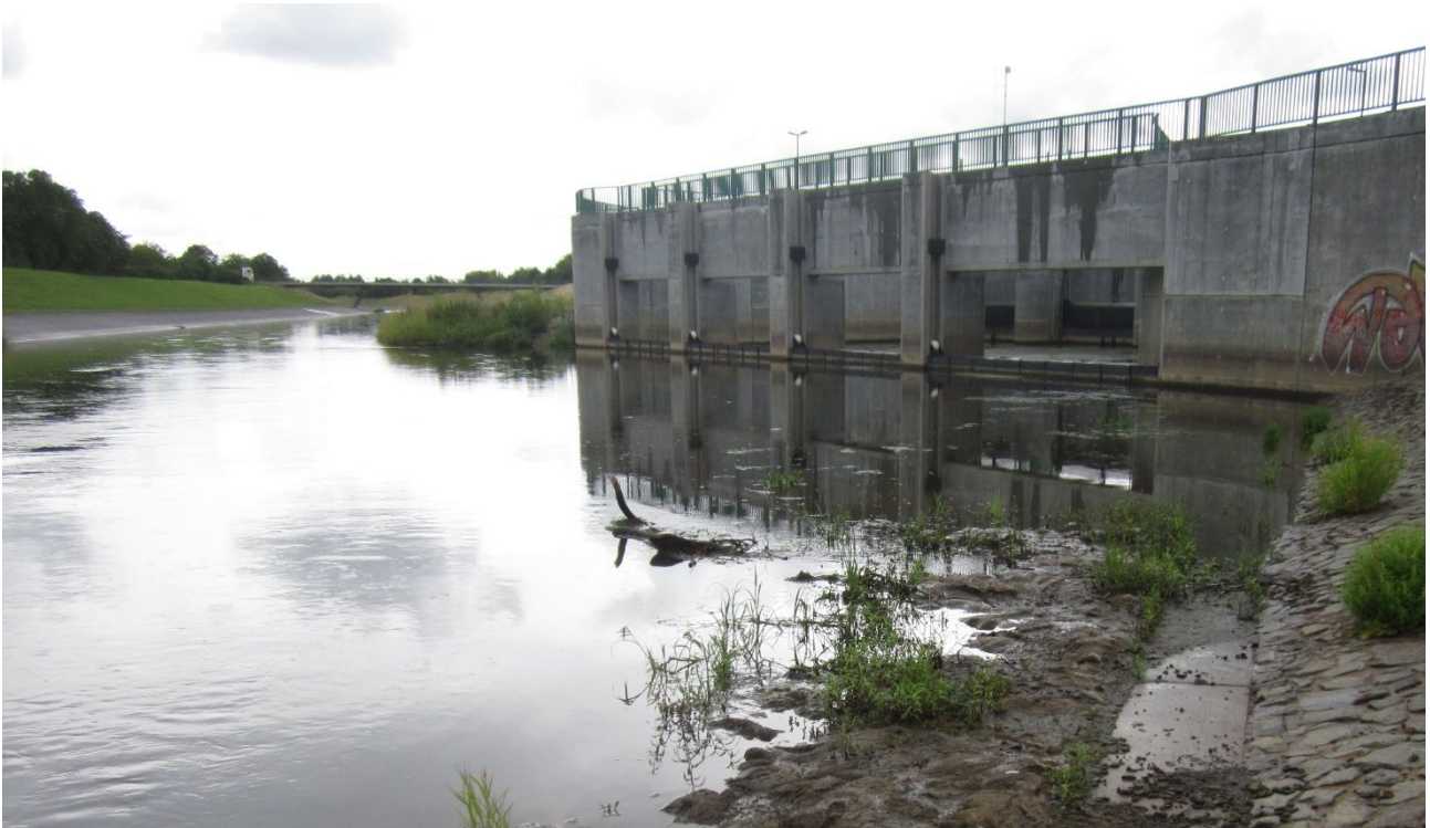
Figure 9. Inflow structure into the Muldereservoir (Photo courtesy of Martin Schultze, Helmholtz Institute).
