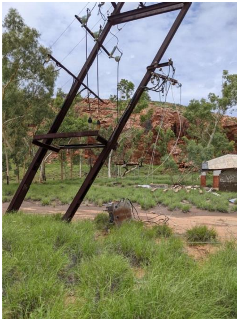
Figure 2: Transformer on Ground
