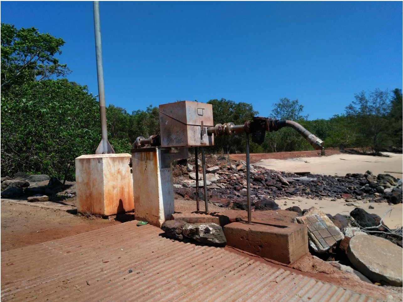
Figure 1. Milikapiti (Snake Bay) barge landing diesel fuel fill point, historical picture.
