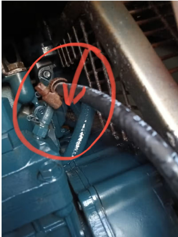
Damage to Line 1
