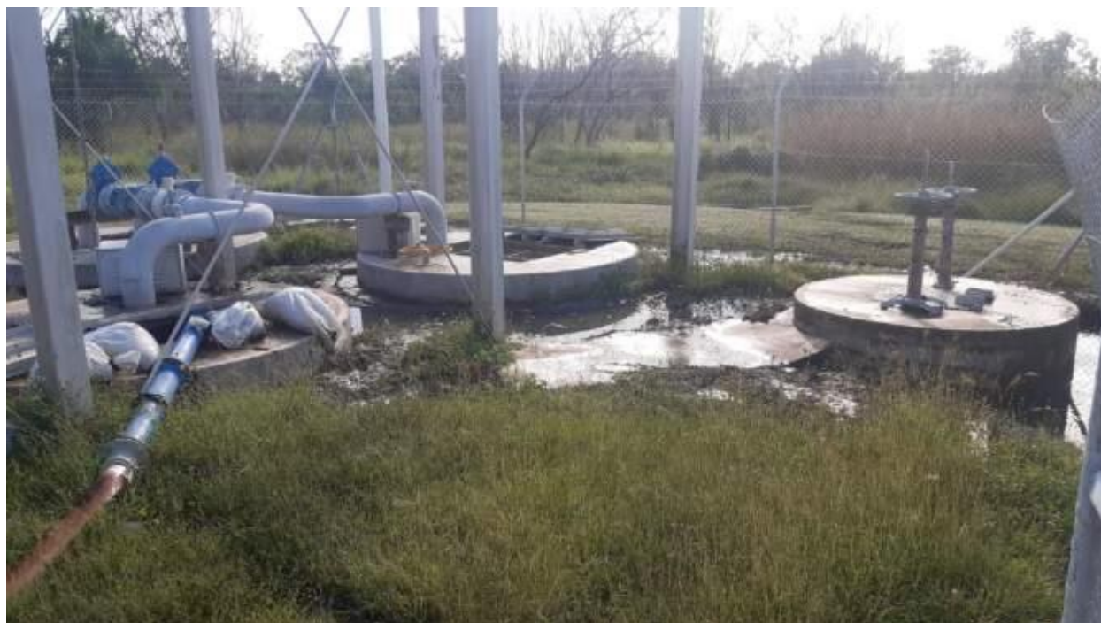
Figure 3: Overflowing Due to Pump failure
