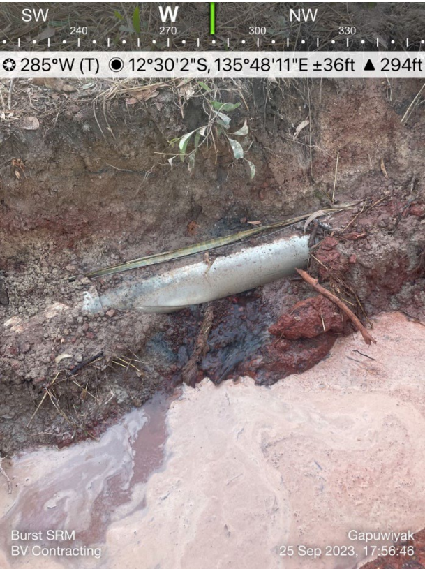
Photo 1. Leak in 150mm sewer rising main
