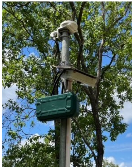
SWTG2 WDL 249 Compliance Point, telemetry station
