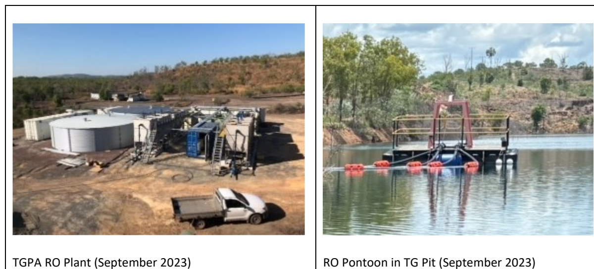
Photo 1-1 TGPA Reverse Osmosis Plant and Pump Pontoon
