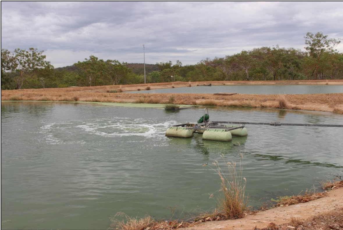
Figure 4: Naiiyu surface aerator in Pond 1 (Power and Water, 2022)
