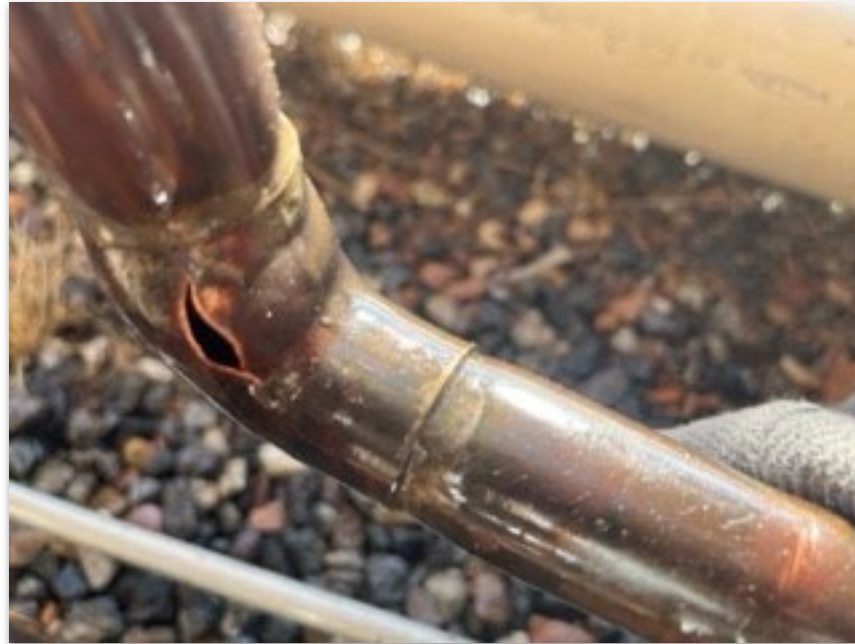
Photo 1. Split in 25mm copper pipe
