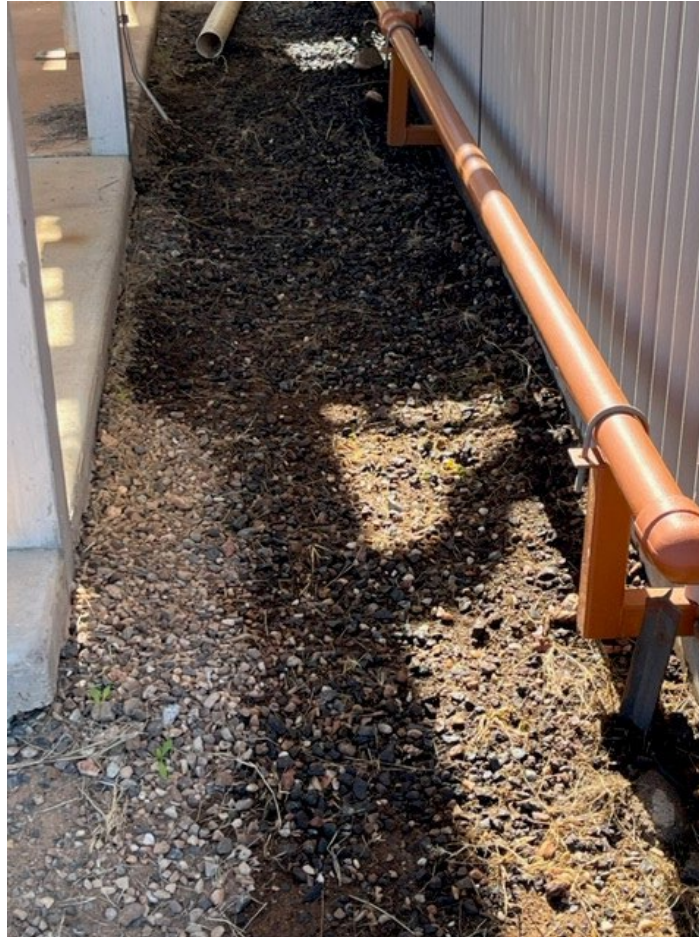
Photo 2. Engine oil spill onto Power-station ground
