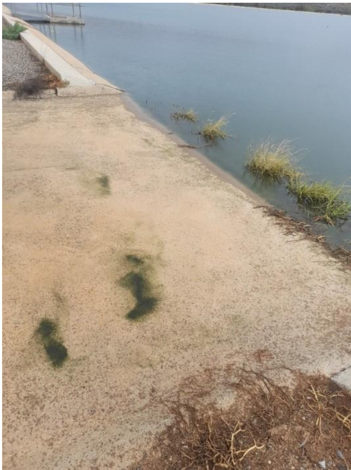
Image 3: Emergency discharge spillway at pond C3, showing that the overflow has ceased. Taken 26/03/2024.
