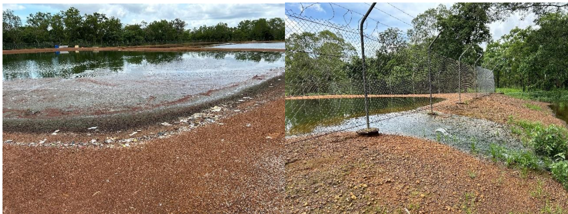
Annual overtopping of Wurrumiyanga waste water ponds observed in February 2024
