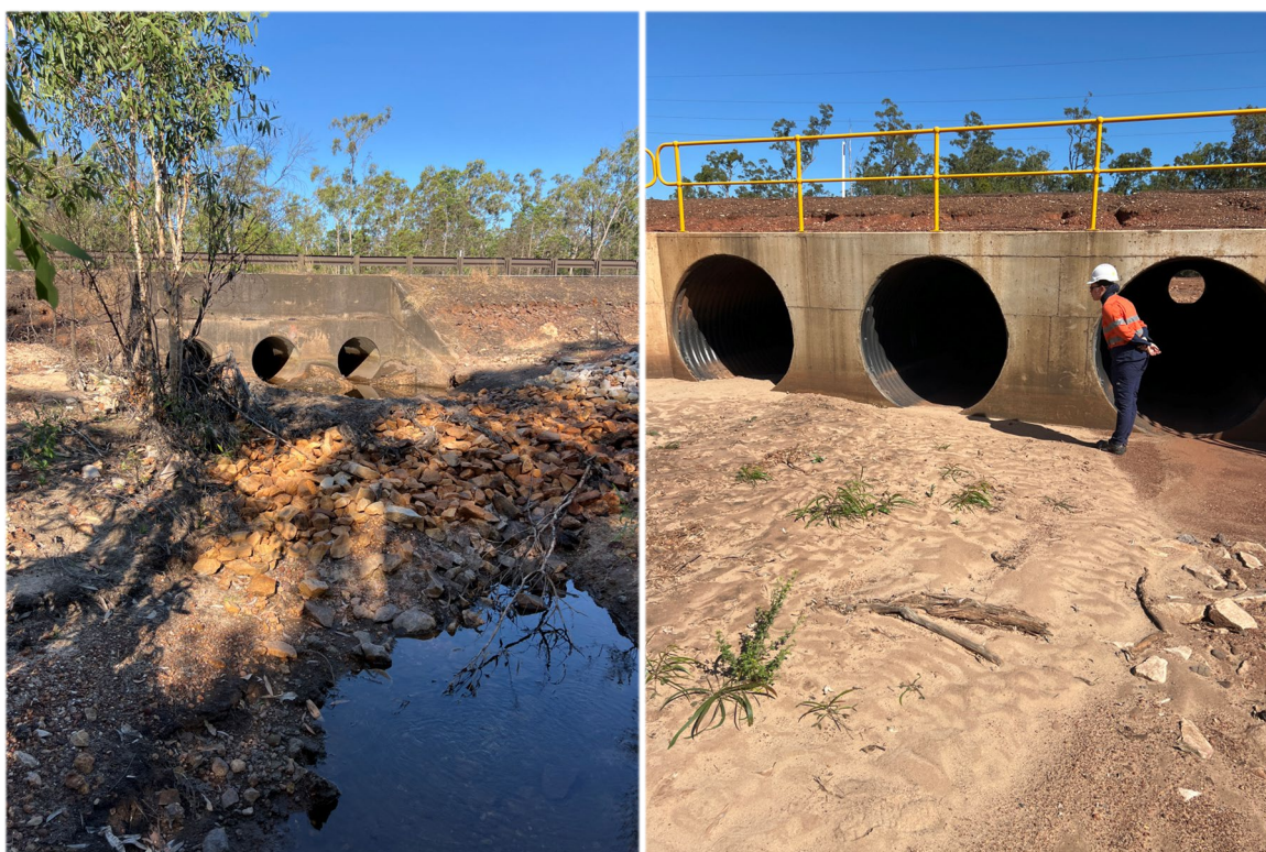
Figure 16 Two of the 41 existing culverts under Rowell Highway immediately adjacent to the proposed pipeline alignment.
