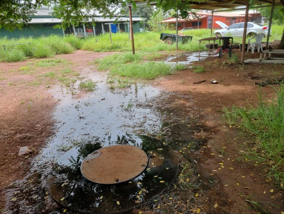
Figure 2. Spill coming from access chamber 4/7.
