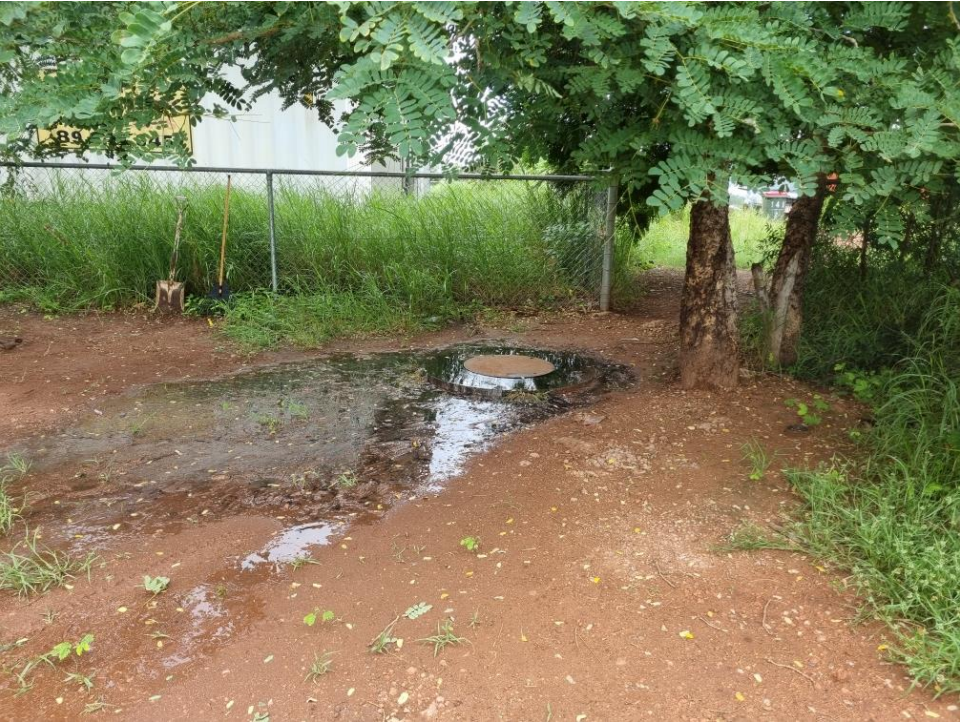
Figure 1. Spill coming from access chamber 4/7.
