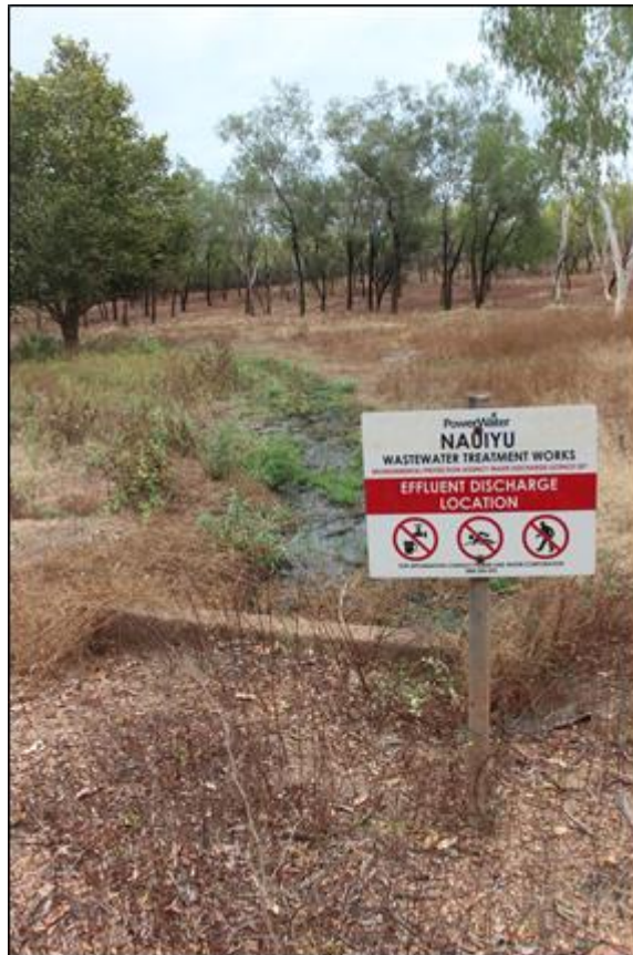
Figure 41. Effluent warning signage at Nanyi DP (PWC, 2022)
