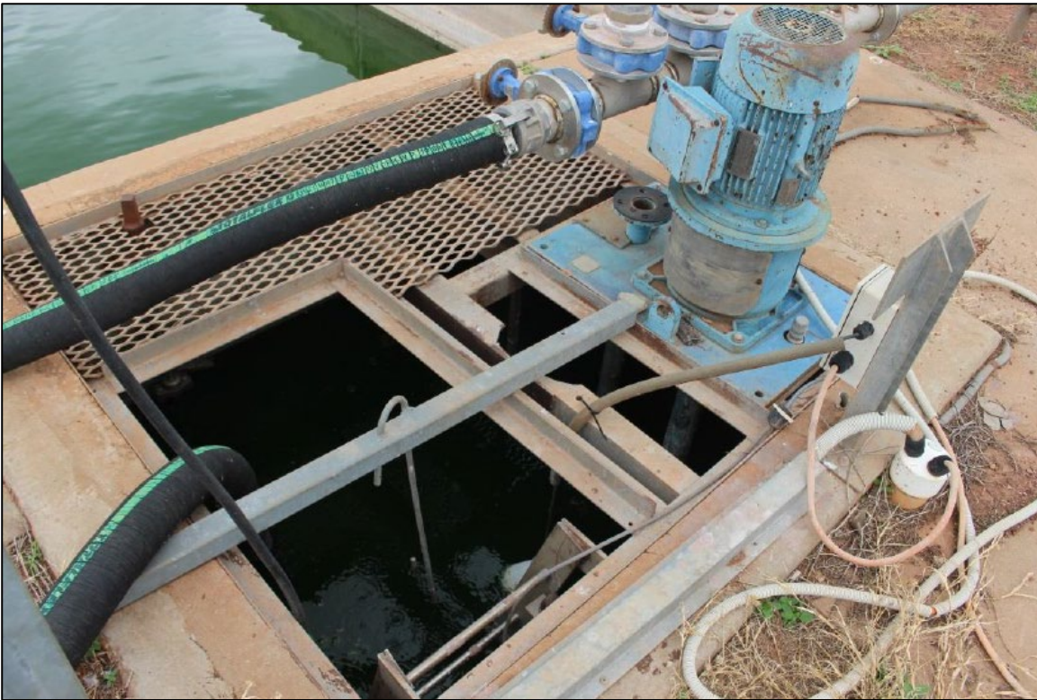
Figure 5: Irrigation pump (PWC 2018)
