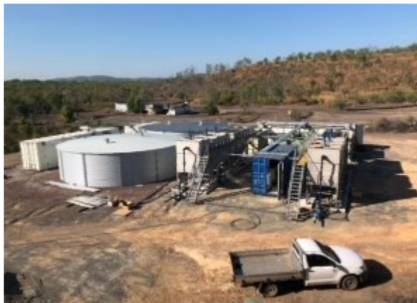
TGPA RO Plant (September 2023)
