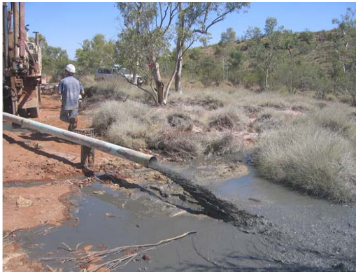
Black water flow from 83 metres at drillhole TMRC41
