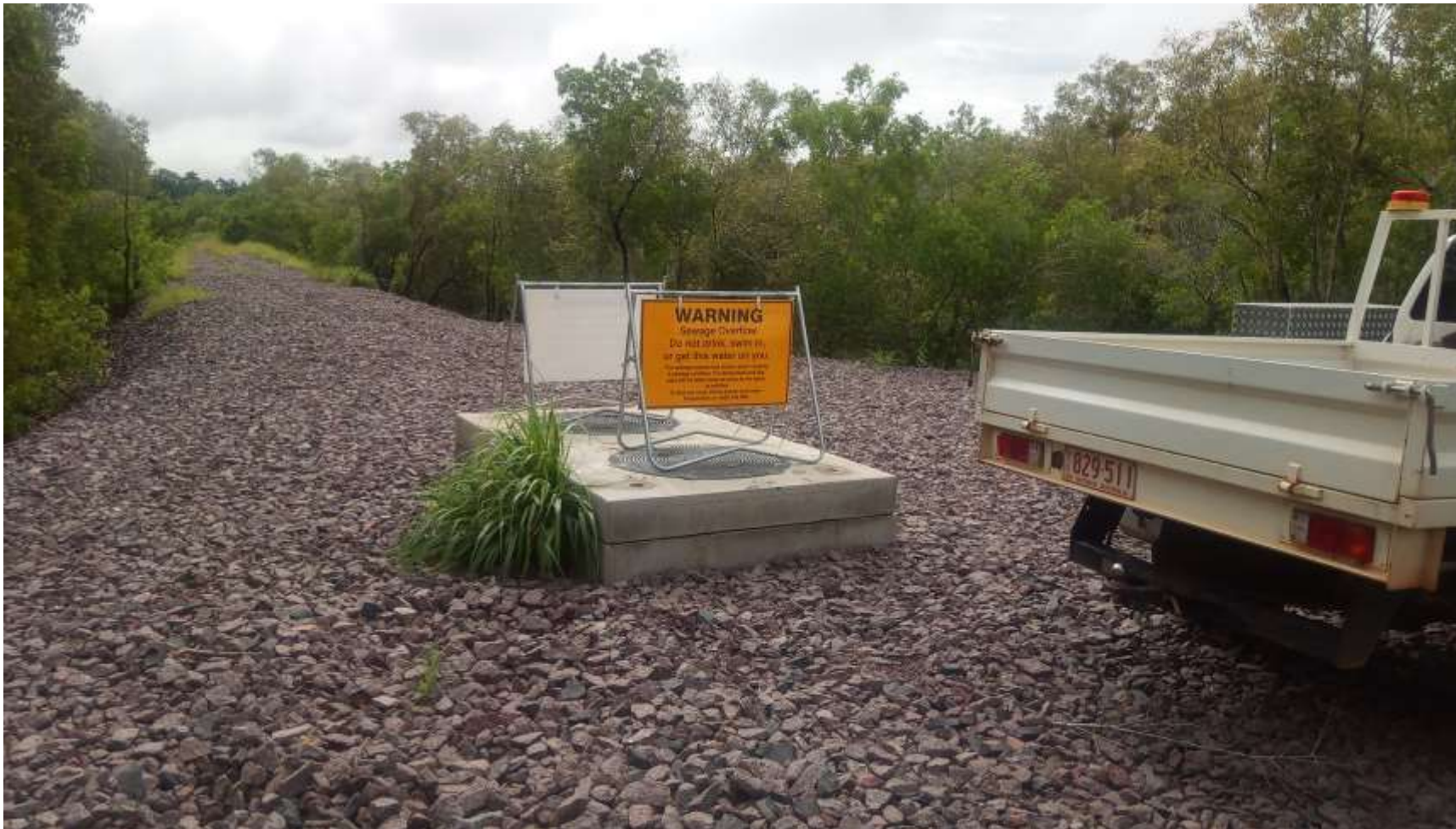
Lakeside Drive and Rapid Creek Road SPS Photo – Warning Signs
