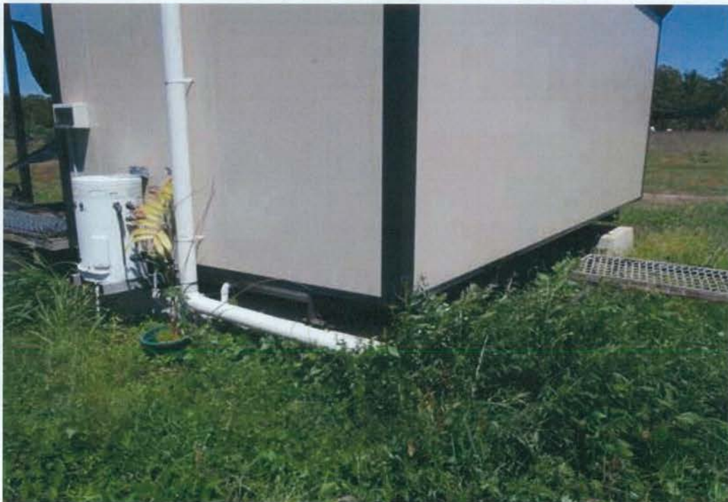
Photo 14: View of pipe work leading to septic system
