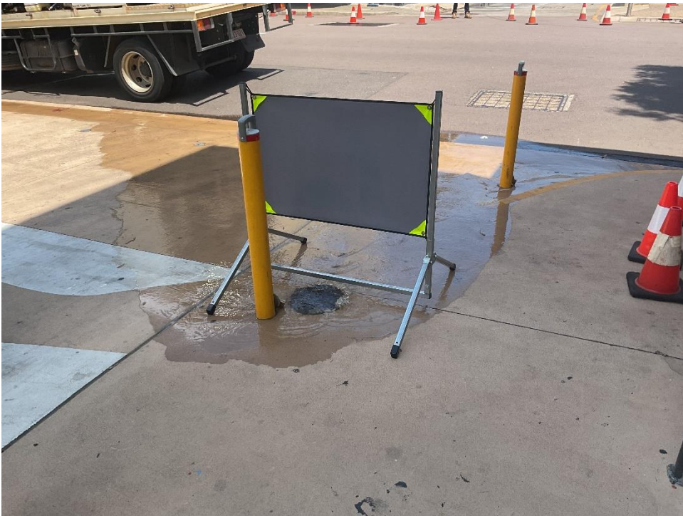
Figure 3 – Discharge point 3 (un-named inspection opening)
