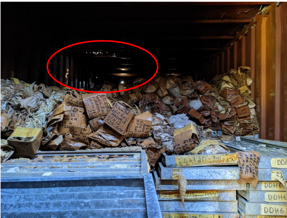
Figure 45. A person can fit their hand in the door gap in container #5 and take a photo of the inside of the container. There appears to be holes in the roof of the container letting light in
