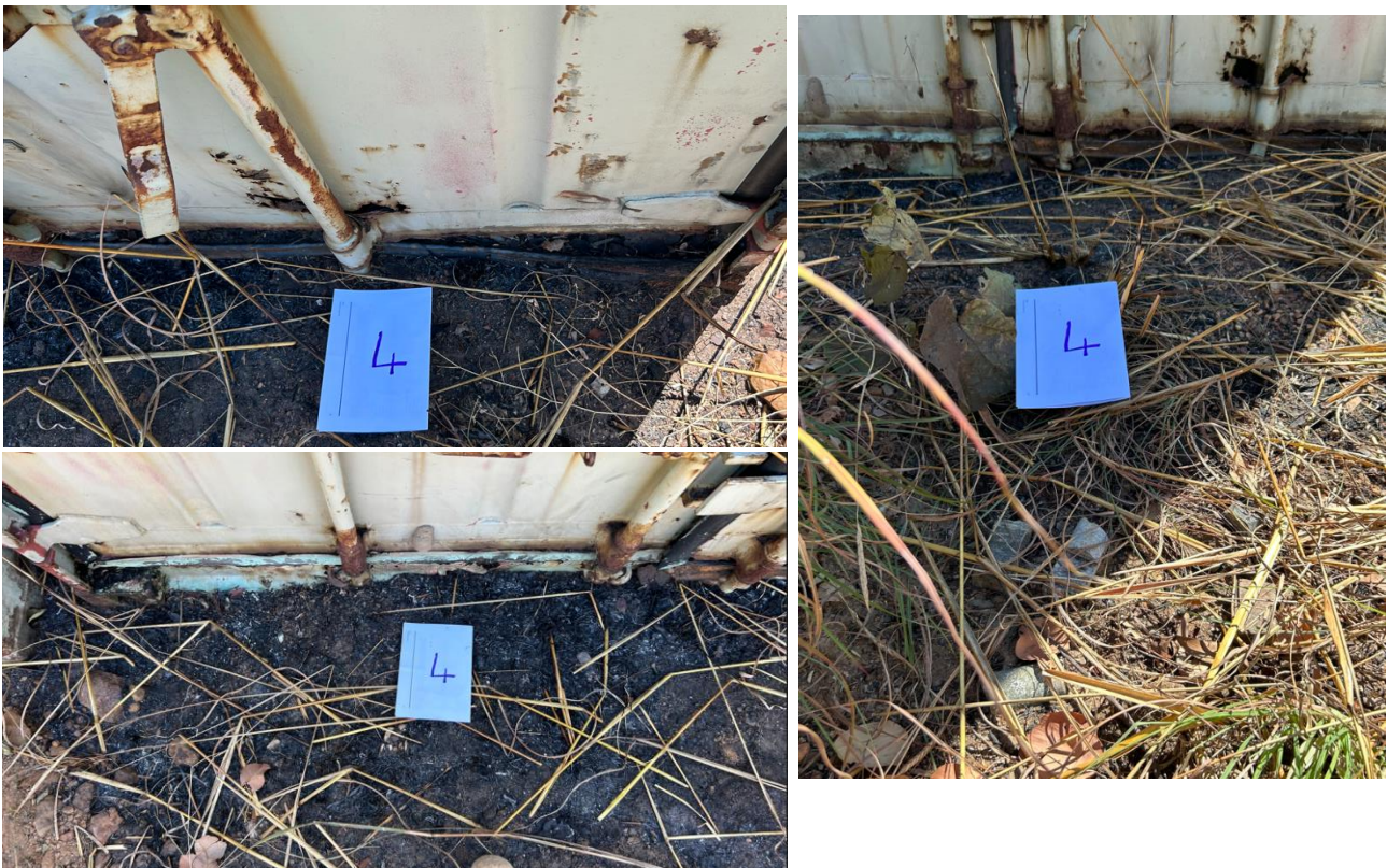
Figure 39. Close up photo showing degradation along bottom of container 4 door. Burnt looking debris is present and a old, rusted oil can is nearby. Broken core samples can be seen in the foreground.
