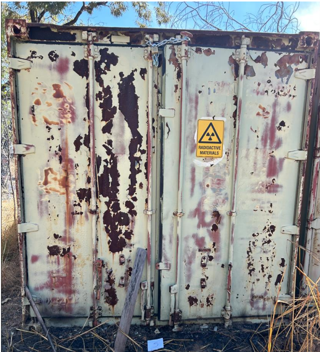
Figure 42. Photo showing radioactive material label and chain and lock on the top of shipping container 5 door. The door of shipping container 5 can't close properly and there is a gap of about 5-10cm where the doors close. Burnt material can be seen in front of the door of shipping container on the ground.
