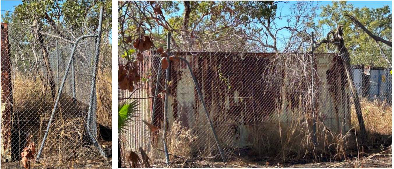
Figure 18b. Close of the corner pole damage and tree branches on the right side of fence, side view of the right side of the fenced enclosure. The fallen branches on the fence could be attributed to the broken tree on the inside the enclosure
