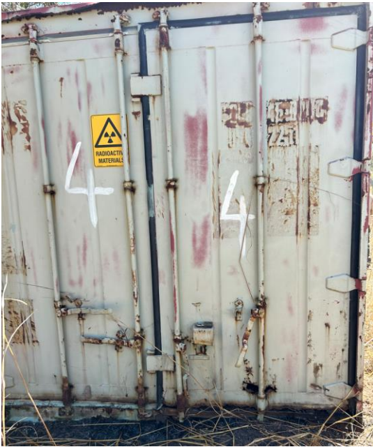
Figure 38. Photo showing shipping container 4 door and radioactive material warning label. The door has not been chained or locked due to difficulties doing this (likely due to door mechanisms seizing due to rust and environmental conditions). Rust degradation can be seen along the top and bottom edges of the door
