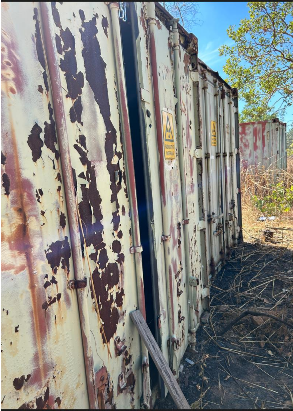
Figure 44. Close up of the door gap on container 5
