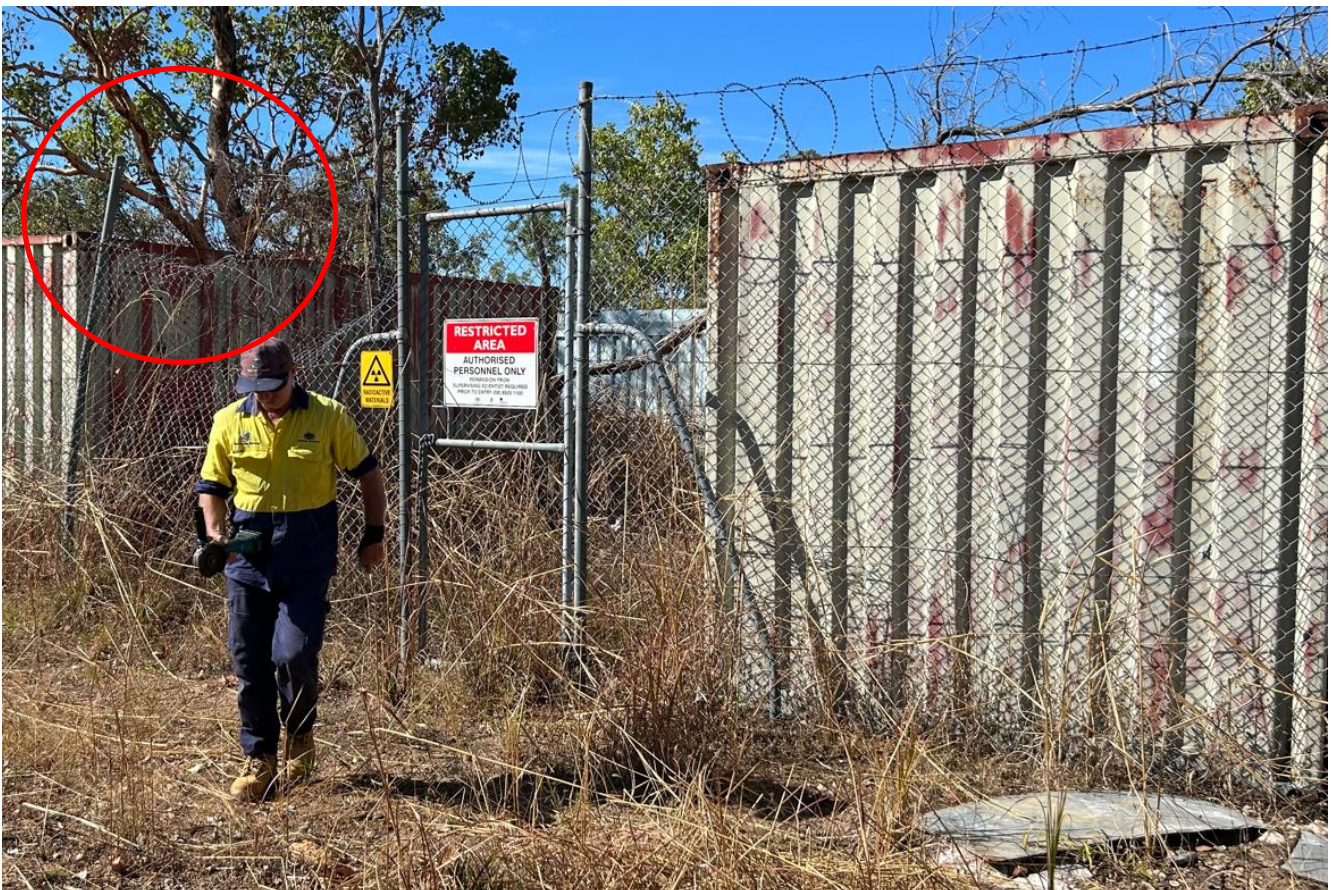
Figure 19. Photo showing gate secured with chain and padlock, restricted area and radiation warning signage. Note damage to the fence to the left of the gate with a buckled pole and fencing leaning inwards (circled in red).
