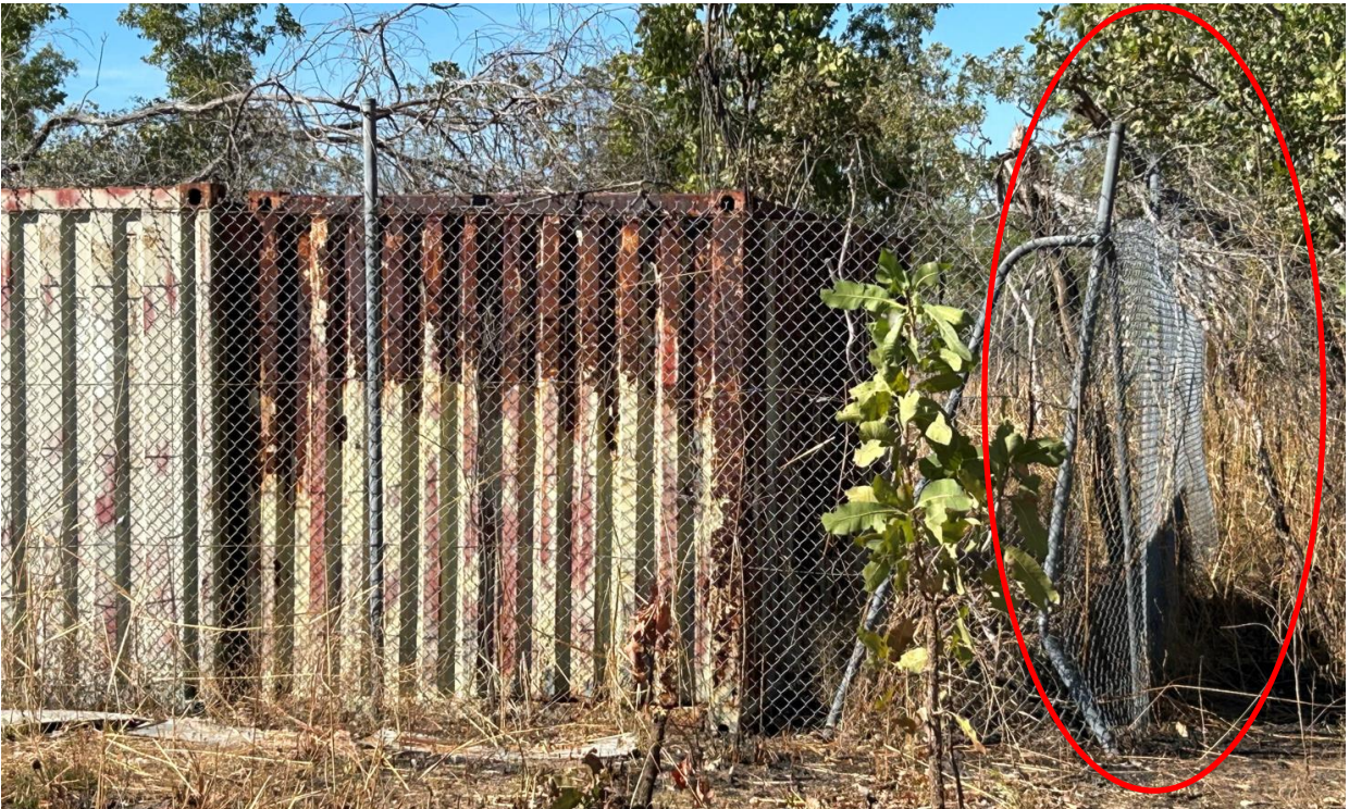
Figure 18a. Close of the damage to corner pole and tree branches on right side of fence. Fallen tree branches can also be seen on top of the shipping containers #4 and #5
