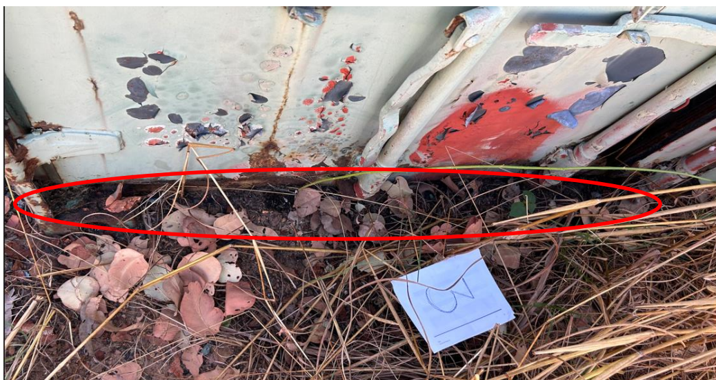
Figure 33. Photo showing closeup of some rust degradation of shipping container door #3.
