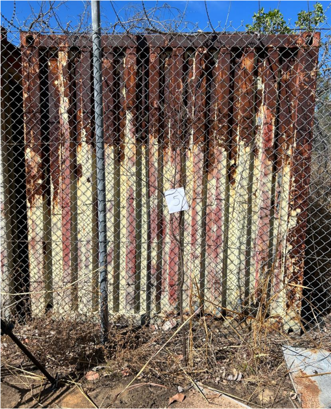
Figure 48. Photo showing condition of end view of shipping container #5. Rust is clearly visible.
