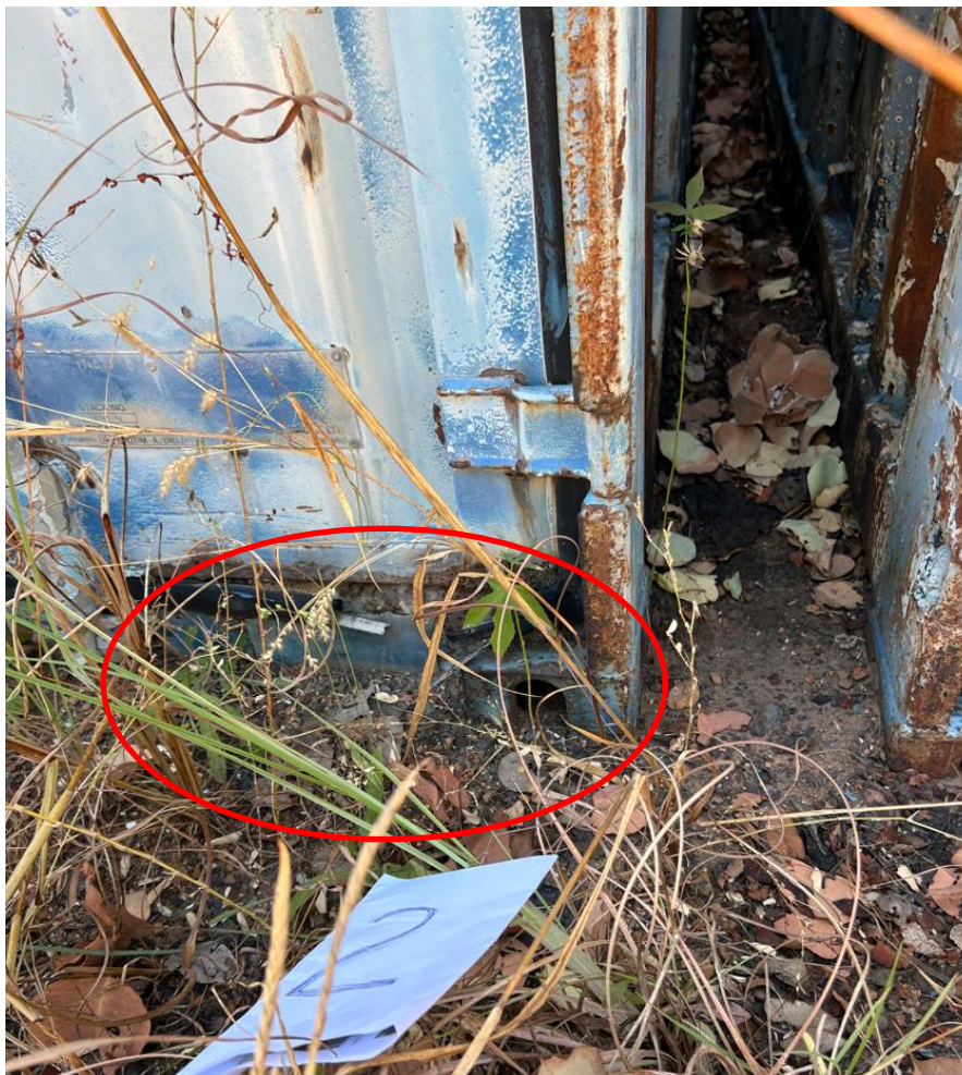
Figure 28. Photo showing some degradation round the bottom door of container #2 and potential sample spill out
