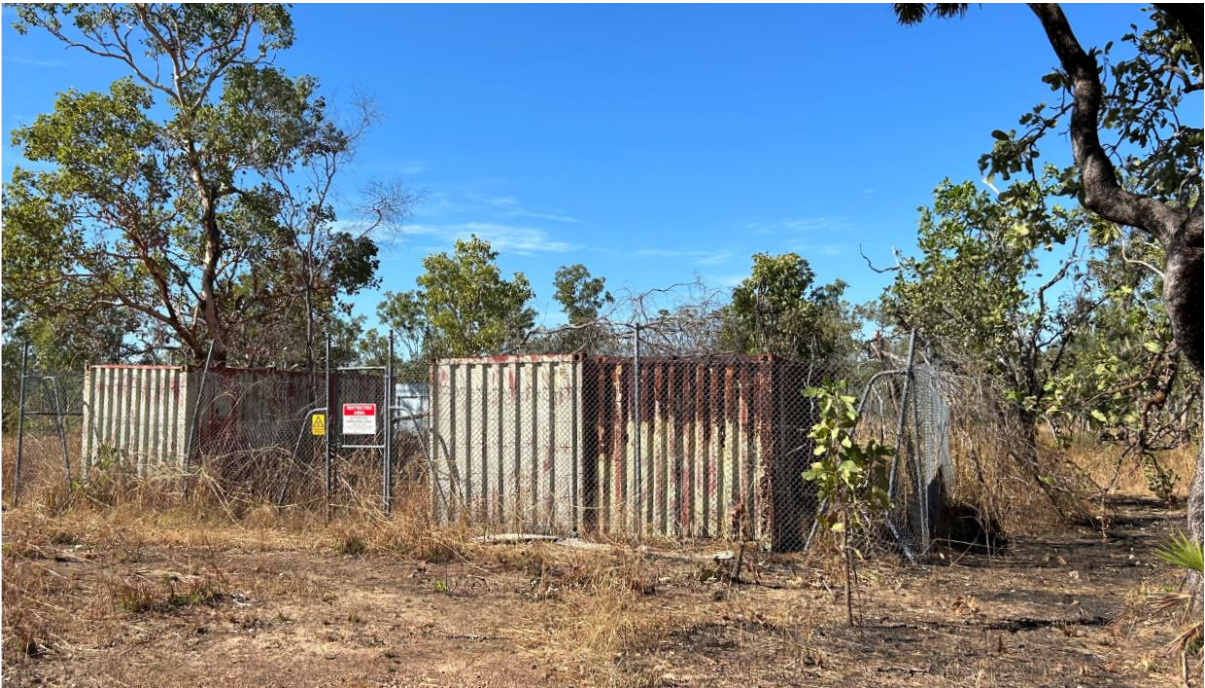
Figure 17. Photo of the secured fenced source enclosure as first sighted. Points of note include the right corner fence damage (bent corner pole) and the tree branches on the right side of the fence.
