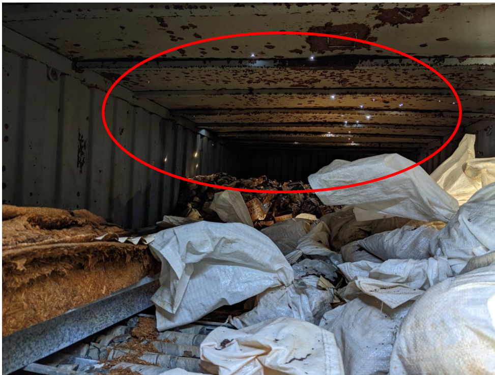
Figure 37. A person can fit their hand in the door gap in container #3 and take a photo of the inside of the container. There appears to be small holes in the roof of the container letting light in
