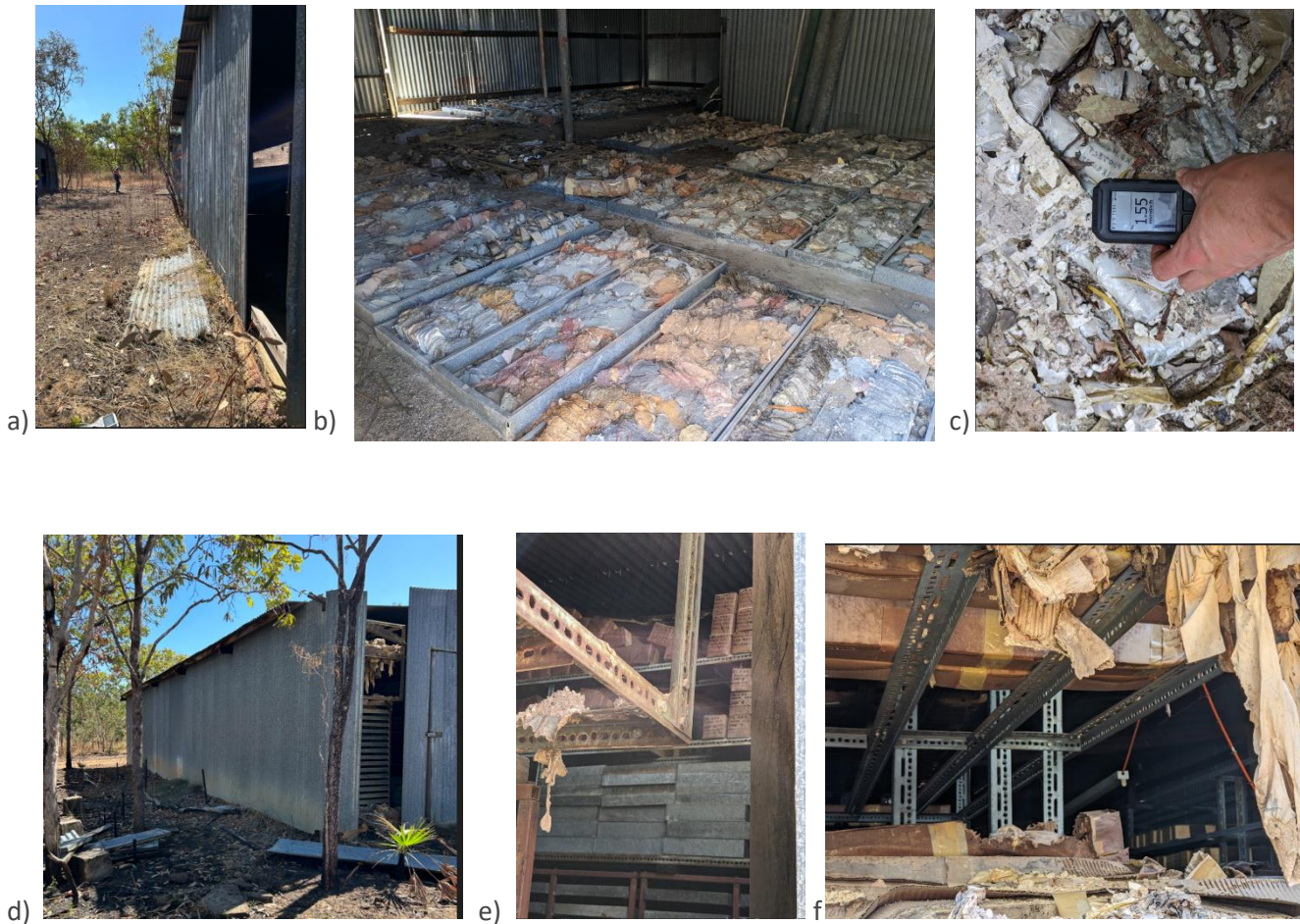
Figure 51a. The sheds are readily accessible due to missing wall and roof panels and are not secured in anyway. b) Photo of inside of shed one showing trays of what appears to be mining cores or samples laid out on the ground. c) Dose rate measurements using a Accurad PRD inside the shed showed reading of 1.55 \mu\text{Sv/h} . d) to f) Shed stacked of sample trays can be seen in shed 2 with trays also seen on the ground in the left of the photo.
