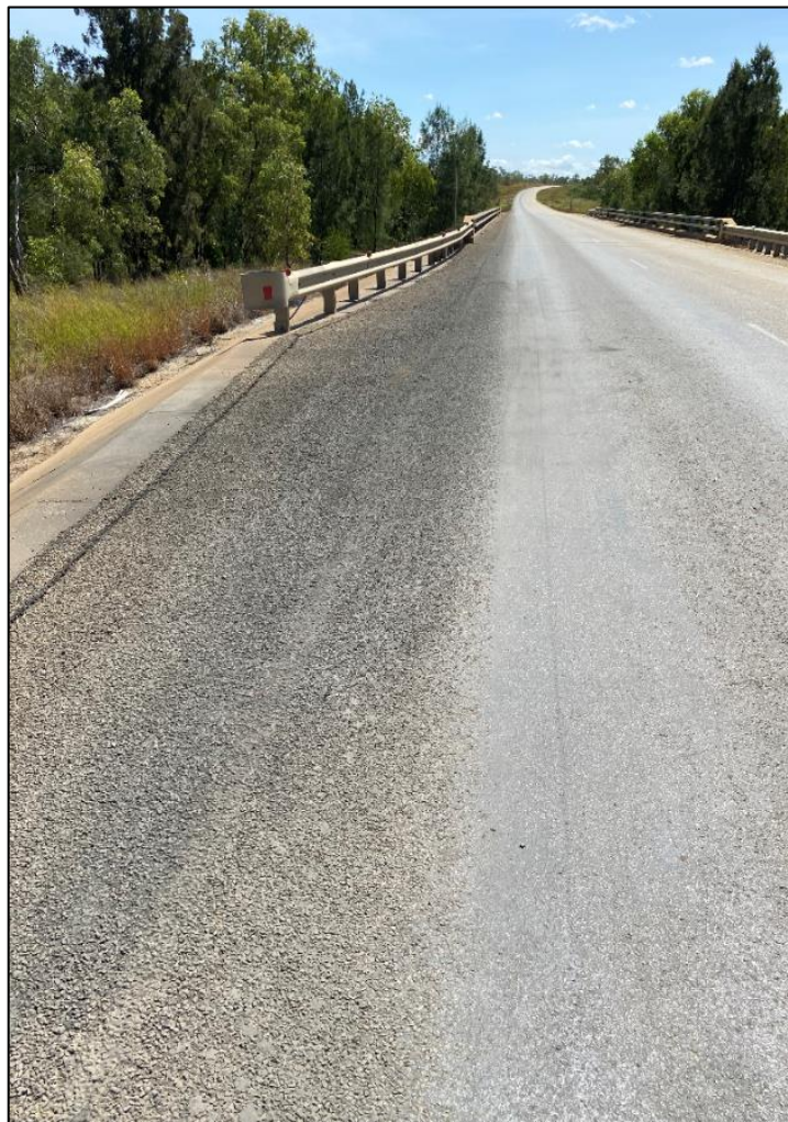
Figure 2: The Carpentaria Highway north bound approach to the Barney Creek Bridge (spill location).
