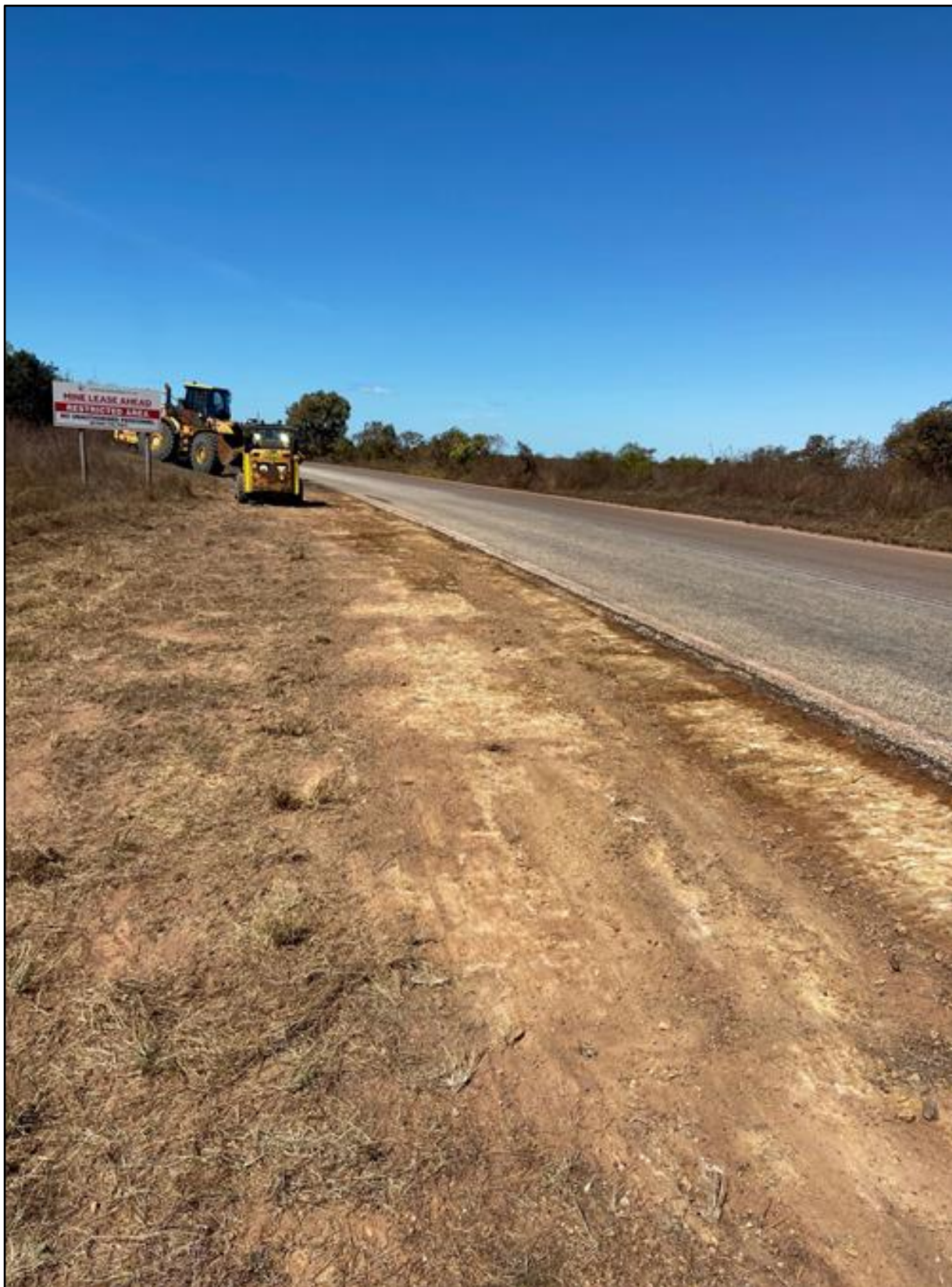
Image 4: During remediation, a bobcat was used to remove all potentially contaminated surface material from the roadside adjoining the incident location.
