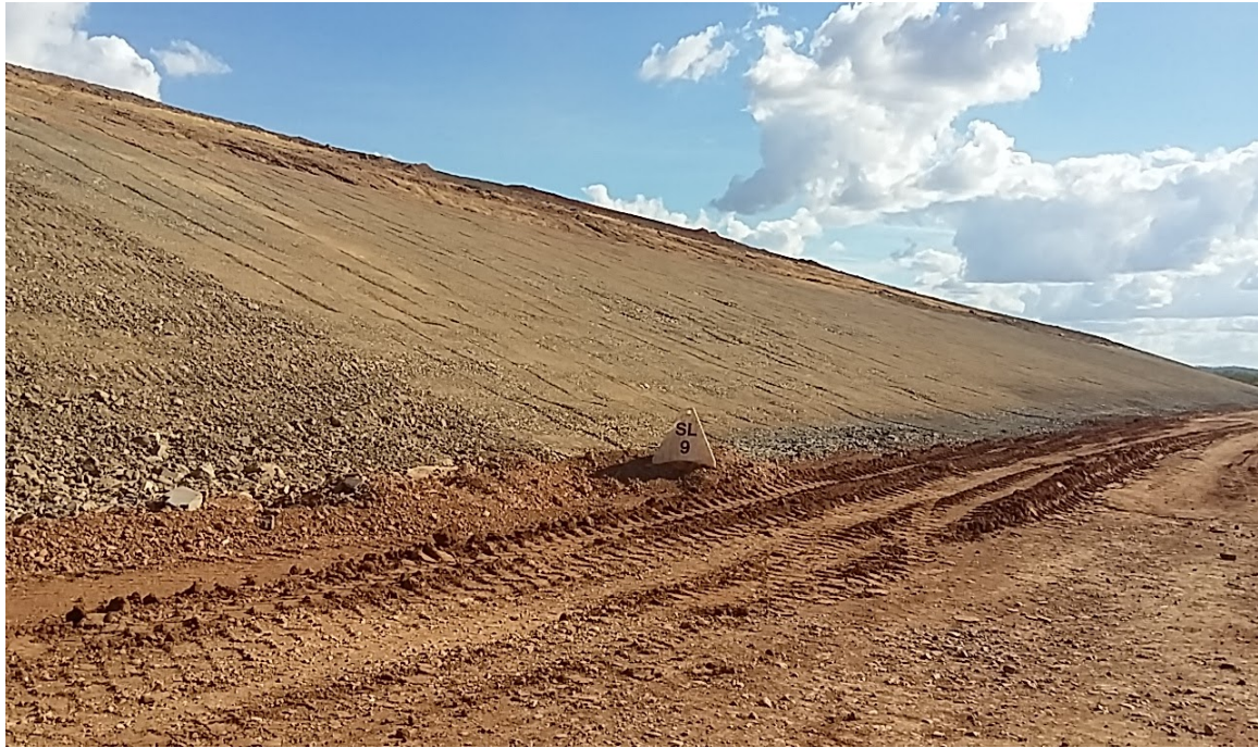
Figure 4 - Rolled shale and alluvial materials on the NOEF
