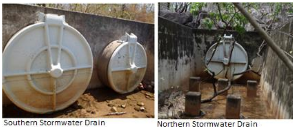
Figure 1: CIPS discharge outlets
