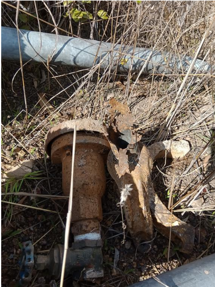
Appendix B – Photographs of the old highly corroded air valve and the newly fitted air valve.
