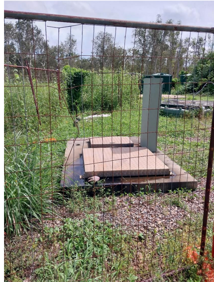
Figure 2. Overflowing SPS within the privately owned WWTP. Source: C. Briscoe – Power & Water
