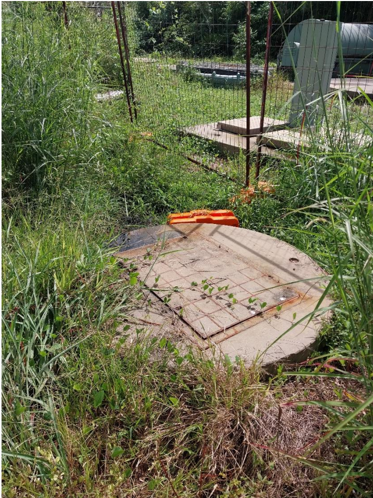
Figure1. Power & Water Manhole cover 1/1. Source: C. Briscoe
