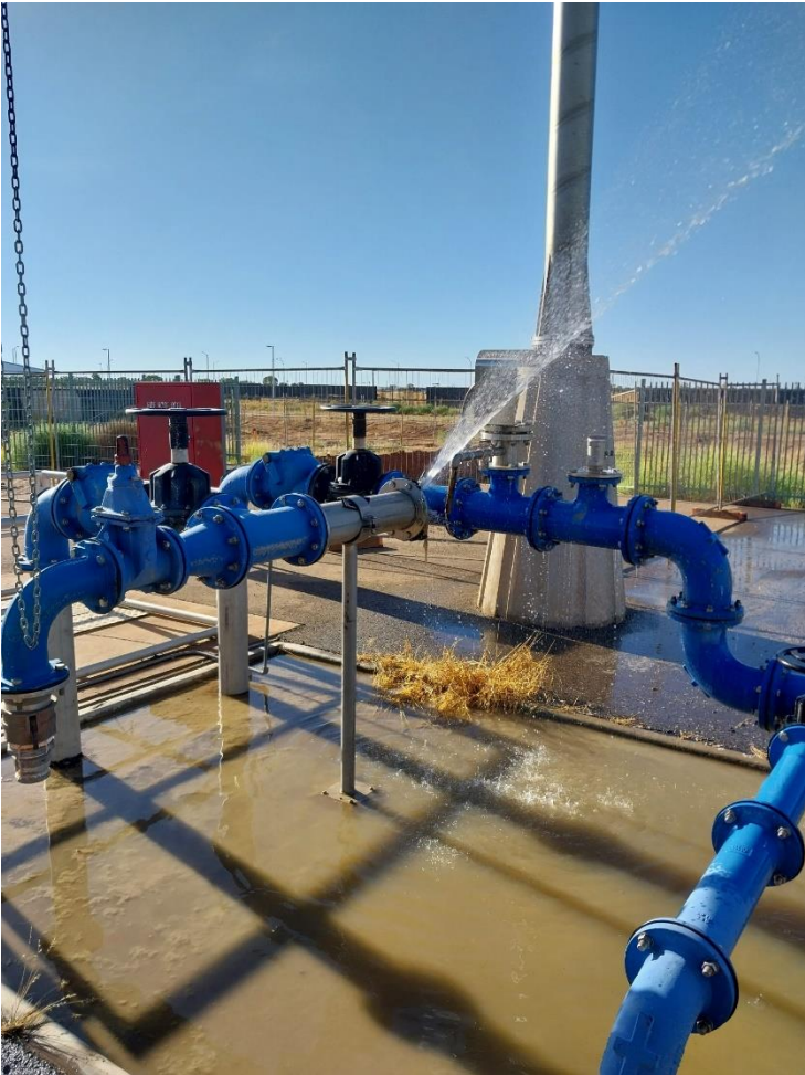
Image 2: The manifold with the leaking gasket, spraying sewage.
