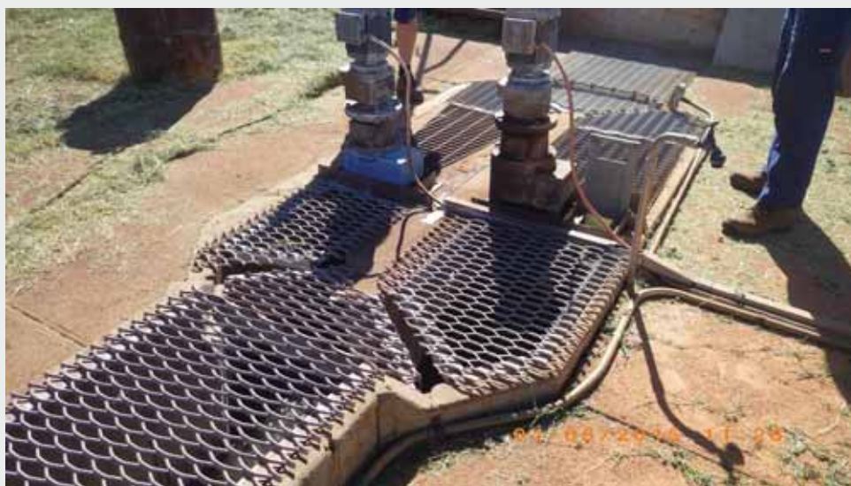
Tennant Creek Sewage Treatment Plant
