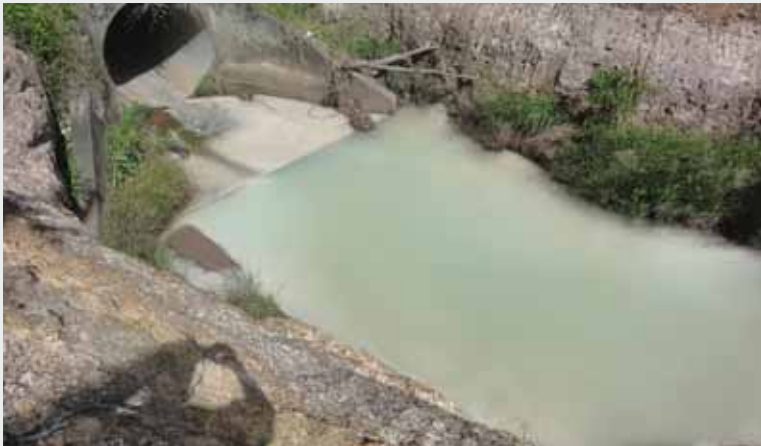
Concrete washing into waterway
