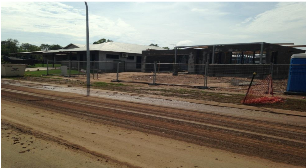
Figure 3-9: Mud from building site posing traffic hazard on public road (NT EPA 2014)
