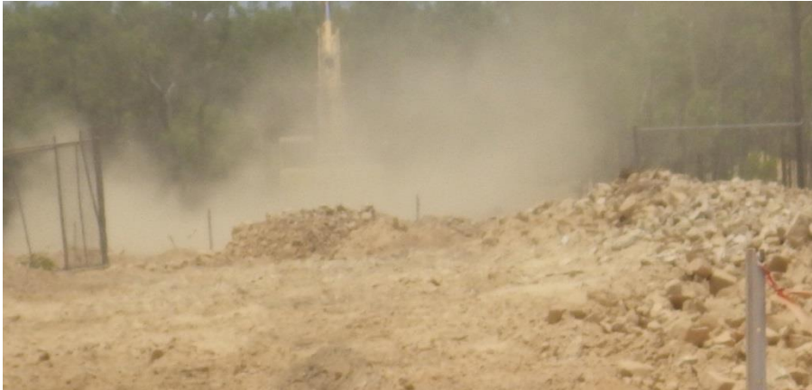
Figure 3-13: No dust control measures in place (NT EPA 2014)
