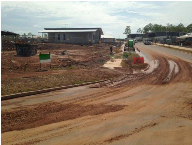
Figure 3-10: Mud from unprotected building sites impacting a public road (NT EPA 2014)
