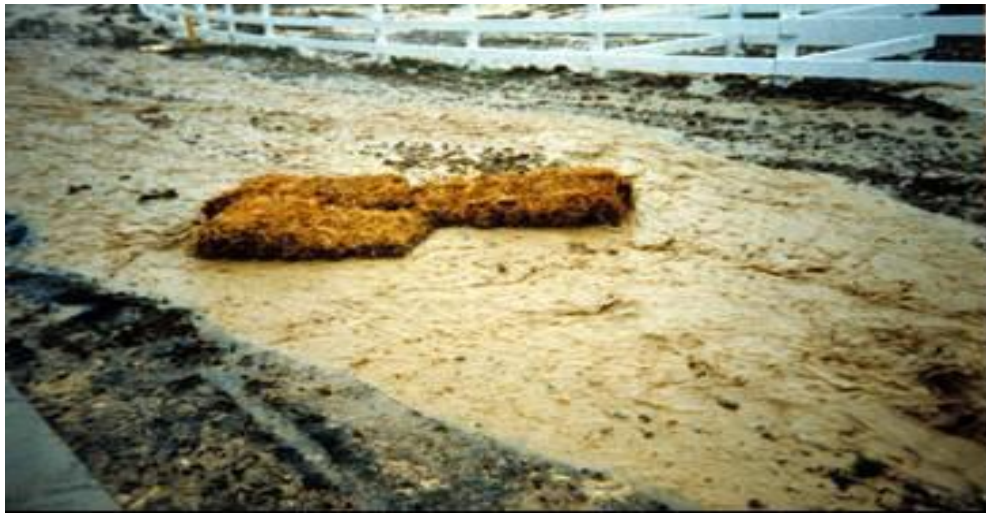
Figure 6-11: Failed hay bale structure bales not staked; catchment is far too big and the barriers are located in a high volume flow path (Environment Canterbury Regional Council)
