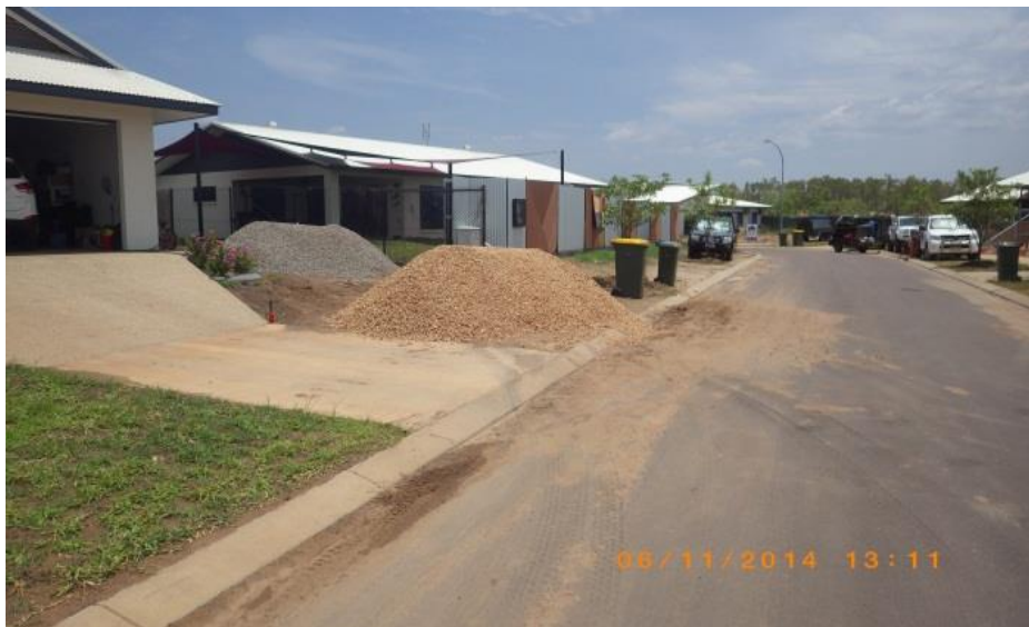
Figure 6-21: Stockpile too close to road as well as being unprotected (NT EPA 2014)
