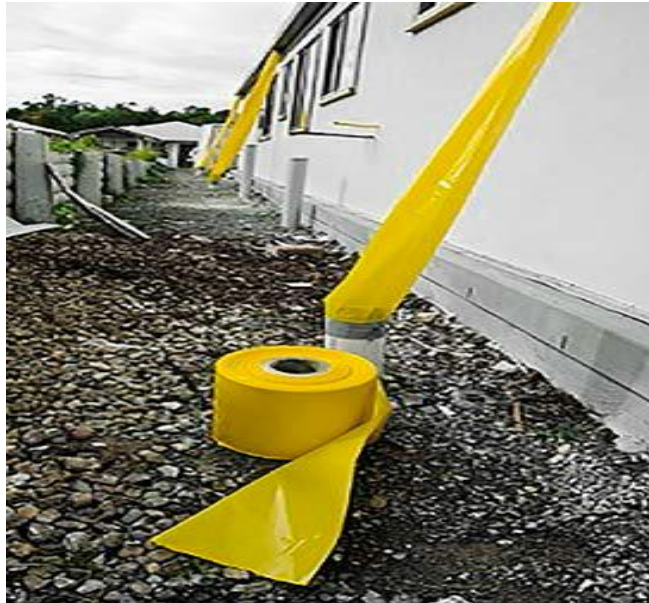
Figure 6-18: Flexible downpipes directed to stormwater entry points (Environment Canterbury Regional Council)
