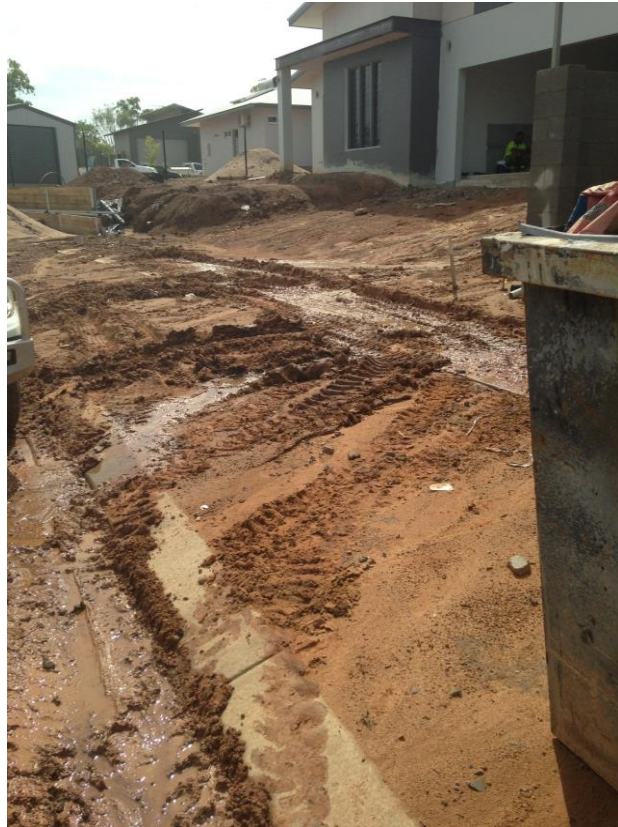
Figure 6-2: No defined entry point causing mud and dirt leaving the site (NT EPA 2014)
