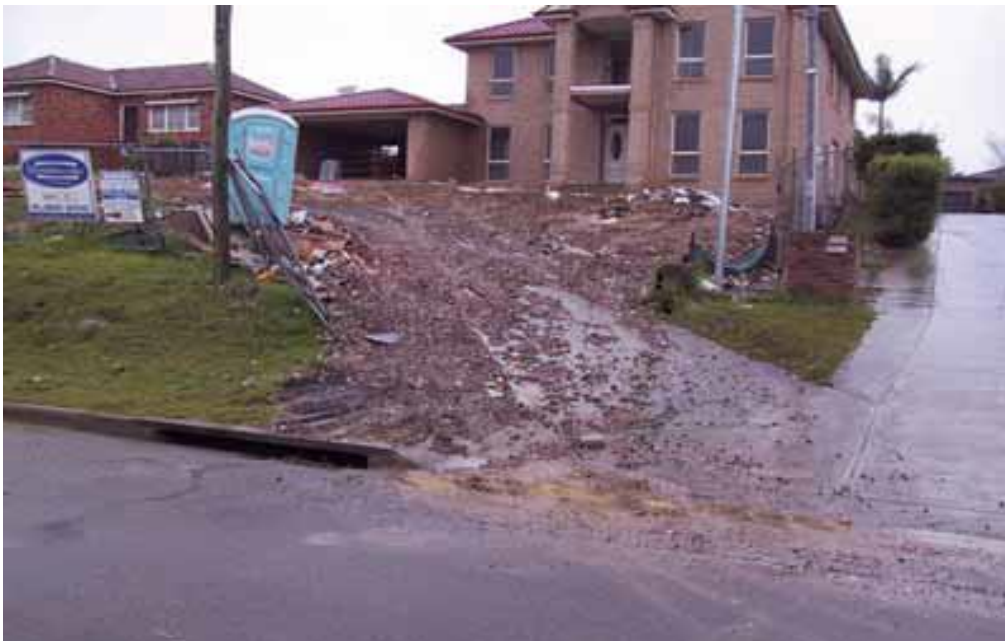
Figure 6-5: Badly managed building site with no controls with nearby unprotected stormwater entry pit (Department of Environment and Conservation NSW)
