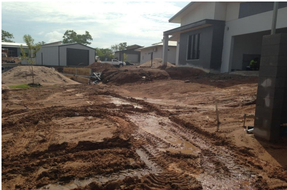
Figure 3-11: Footpath covered by mud posing slip risk to pedestrians (NT EPA 2014)
