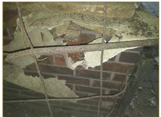
Photograph 6 – Friable paperback vinyl sheeting within the Recreation Club
