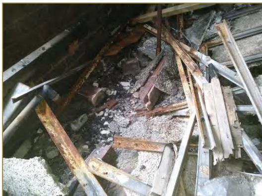
Photograph 5 – ACM sheet debris (including friable materials) strewn throughout the internals of the Recreation Club
