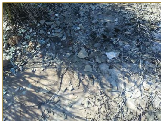
Photograph 16 – ACM debris on concrete pads across the site
