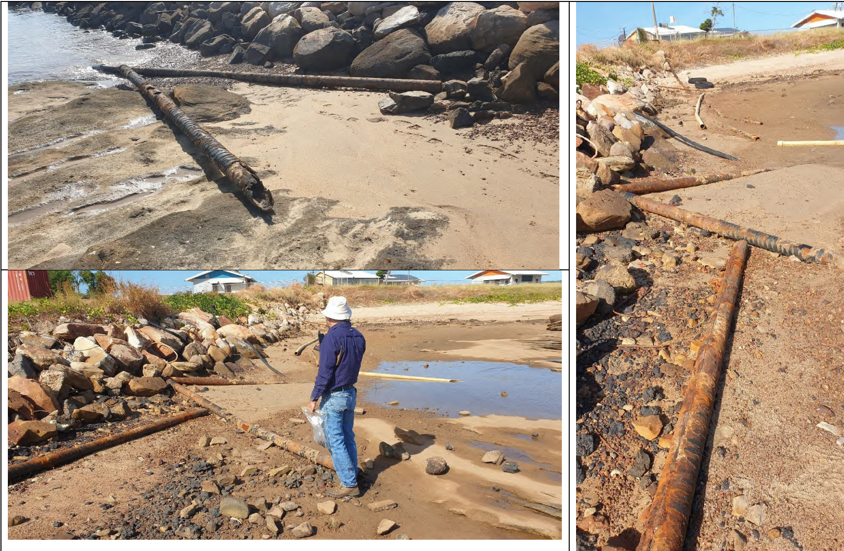
Photo 21 View of broken up cast-iron wastewater pipeline located along western side of Jetty
