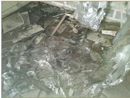
Photograph 7 – ACM sheet debris (including friable materials) strewn throughout the internals of the Recreation Club
