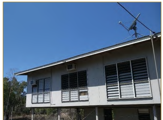
Photograph 30 – Asbestos audit conducted of the South Elevated House (understood to be built pre-2003)
