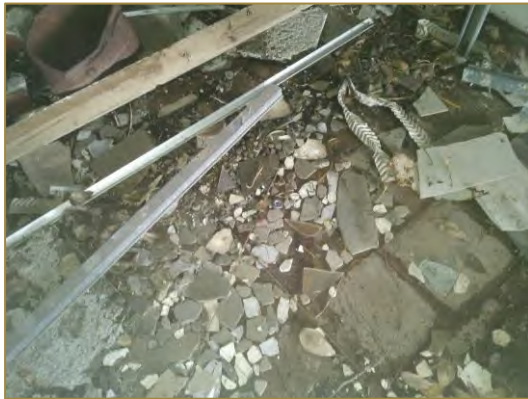
Photograph 3 – ACM sheet debris (including friable materials) strewn throughout the internals of the Recreation Club
