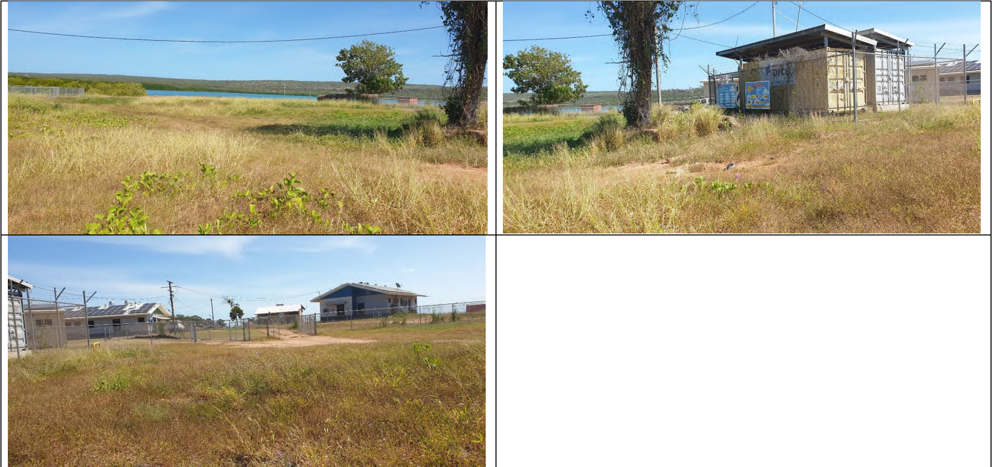
Photo 25 View of generator area
