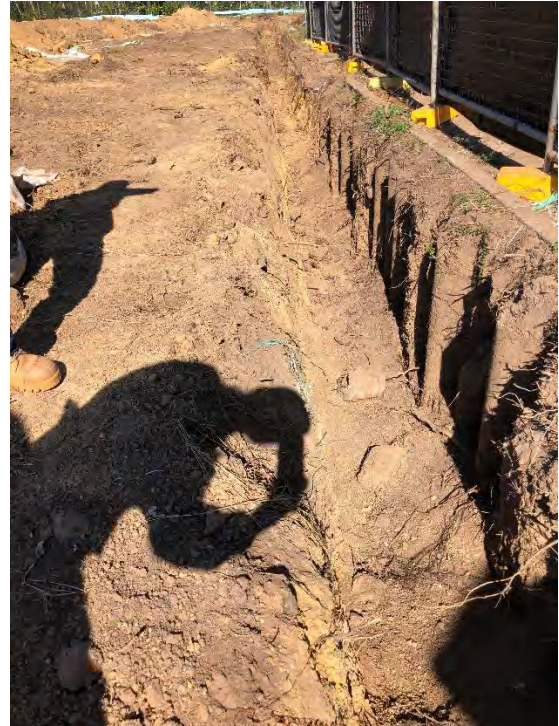
Plate 3: Trenching to remove additional corrugated asbestos fencing, identified along the northern site boundary.
