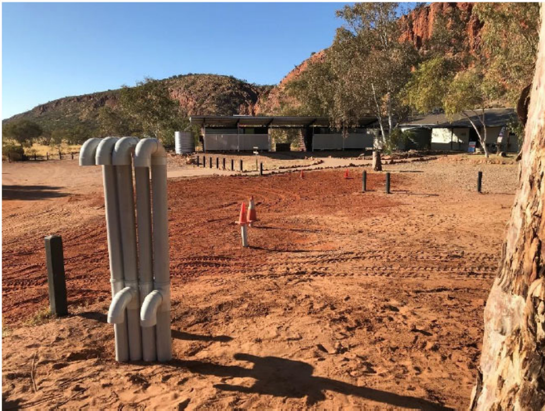
Figure 15. Reinstated Tank Pit Areas – diesel (top) and petrol / Opal (below) (Photos by Low Ecological)
