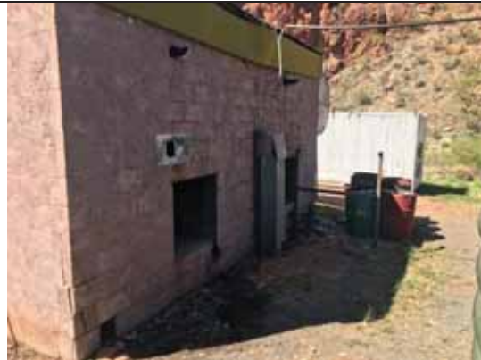
Photo: Back of generator building – note small patches of oil stained soil from crank case breather hoses, and 44 gallon drums stored on ground adjacent to building.
