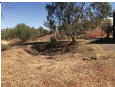
Photo: Old sludge/overflow/storage turkey nest dam – Note thin black plastic liner deteriorated/disintegrating at top of banks. Dry dark odourless composted biosolids present in bottom.
