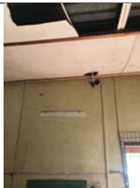
Photo: Broken/damaged wall cladding.
