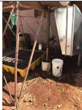
Photo: Catch bucket and bund under diesel tank – note diesel stained soil under.
