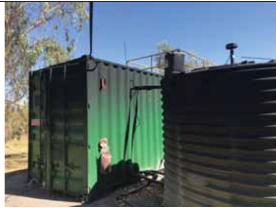
Photo: Soot from generator exhausts deposited on nearby WWTP.
