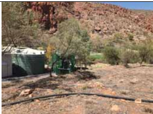
Photo: Wastewater Treatment System – Note stormwater diversion drain upslope, and Finke River waterhole behind.
