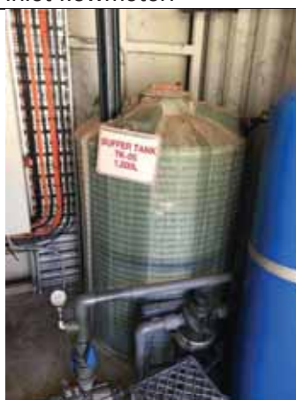
Photo: Evidence of overflow from effluent buffer tank into control/dosing room.
