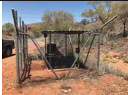
Photo: Bore pump diesel generator in locked enclosure.
