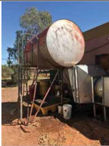
Photo: Above ground diesel storage tank – note stained soil under tank.
