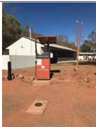
Photo: Unleaded bowser, fill/dip point, vent, and small canopy – Note two vent pipes and unknown filled opening adjacent to bowser.
