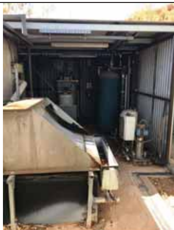
Photo: Old wastewater treatment system - Note liquid still in chemical dosing tank.
