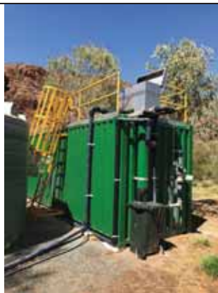
Photo: Inlet pipe and screen into wastewater treatment plant – Note evidence of leakage from inlet flowmeter.
