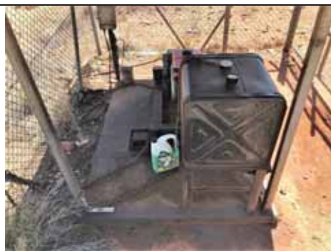
Photo: Generator plinth and diesel tank – note localised oil/diesel staining on and around plinth.
