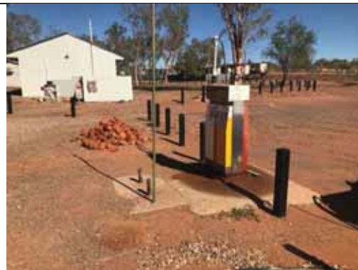
Photo: Diesel bowser, underground tank, fill and dip points, and vent – Note diesel staining on concrete around bowser.
