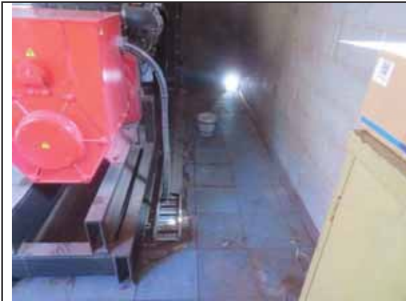
Photo: Generator building floor drains direct to ground/soil outside.
