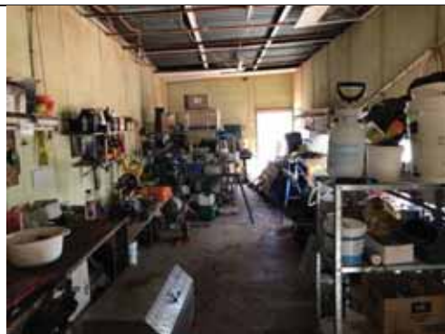
Photo: Main storage shed – wall cladding likely asbestos cement sheetting.
