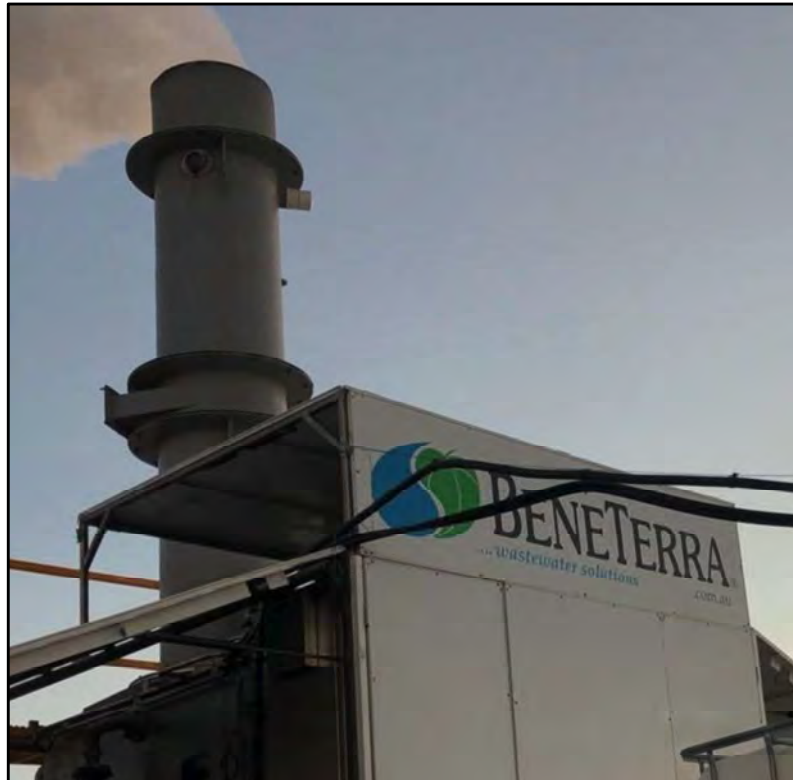
Figure 1: BeneVap Treatment System Stacks
