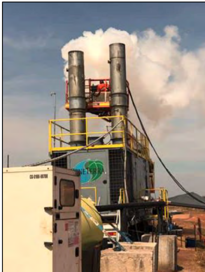
Figure 1: BeneVap treatment system stacks
