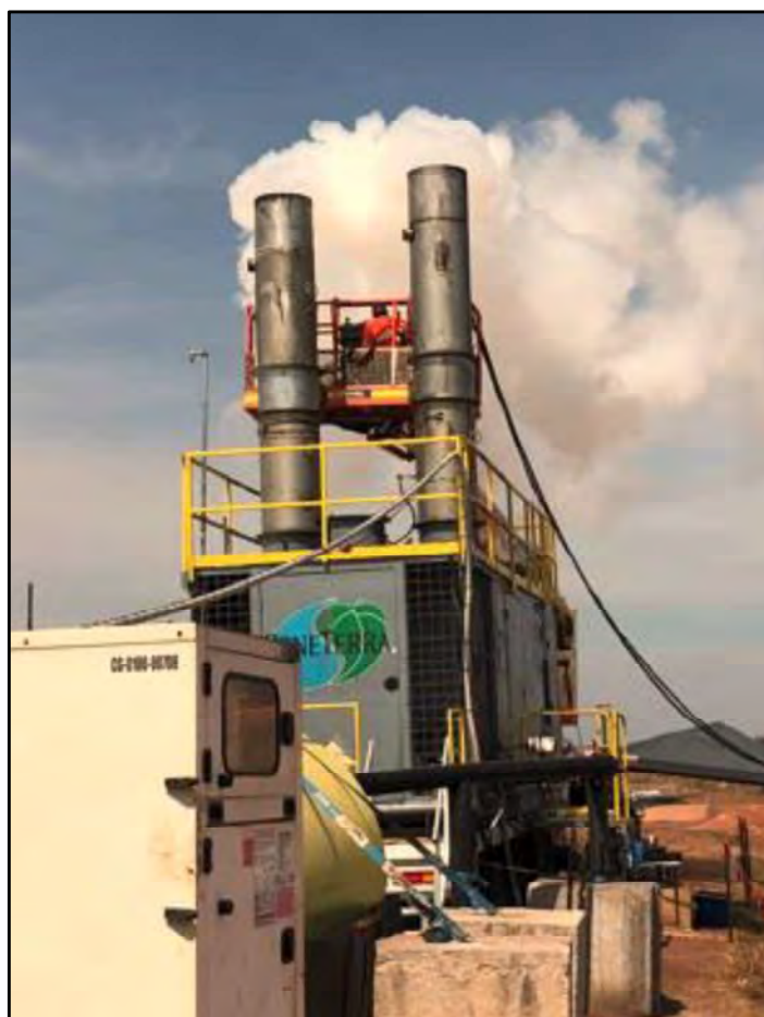
Figure 1: BeneVap treatment system stacks
