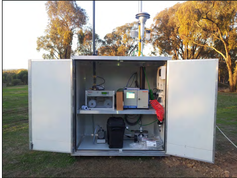
Figure B1 Compact Ambient Air Quality Monitoring Station
