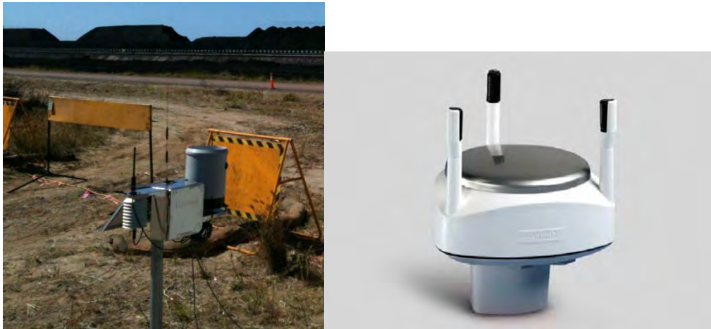
Figure B5 Weather Station and WMT52 Ultrasonic wind sensor
