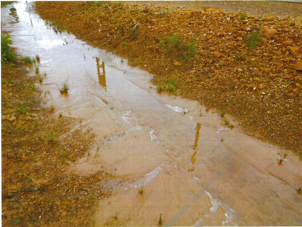
Photograph 5: Earthen stormwater drain located north of the stockpile. Visible hydrocarbon-like sheen visible in water and on surrounding ground surfaces.
