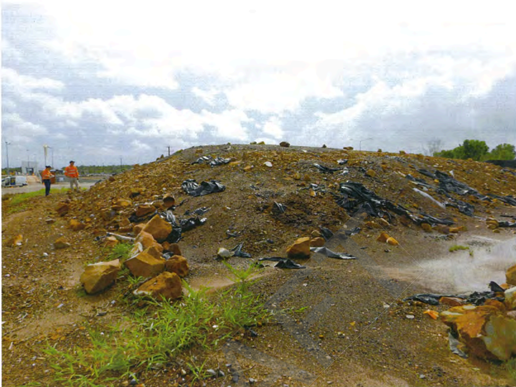
Photograph 1: Stockpiled material facing east. Stockpile is uncovered with no erosion or sediment controls in place.
