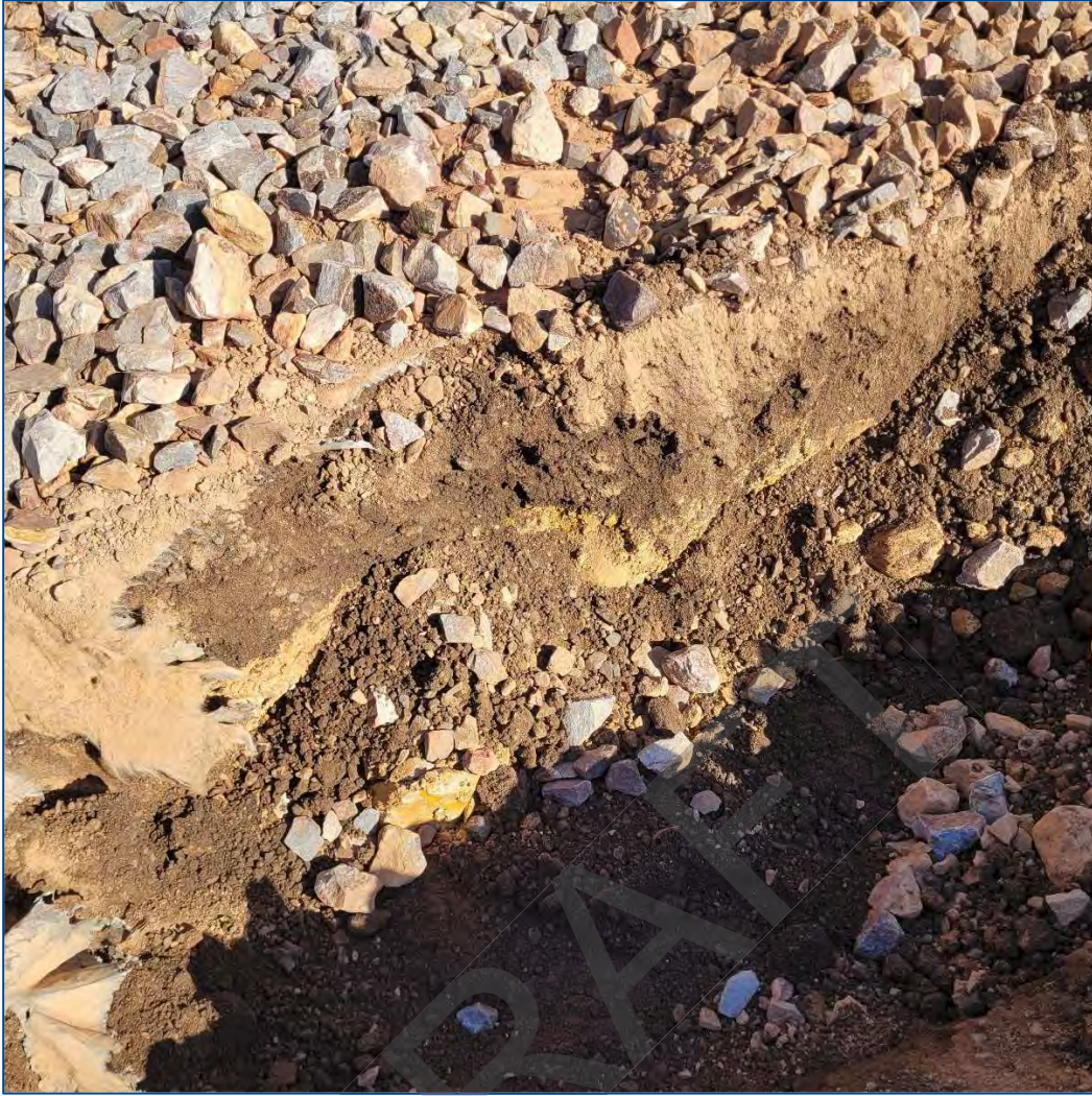
Photograph 5: View of light brown silty sand material underlying dark brown sands in Area 2
