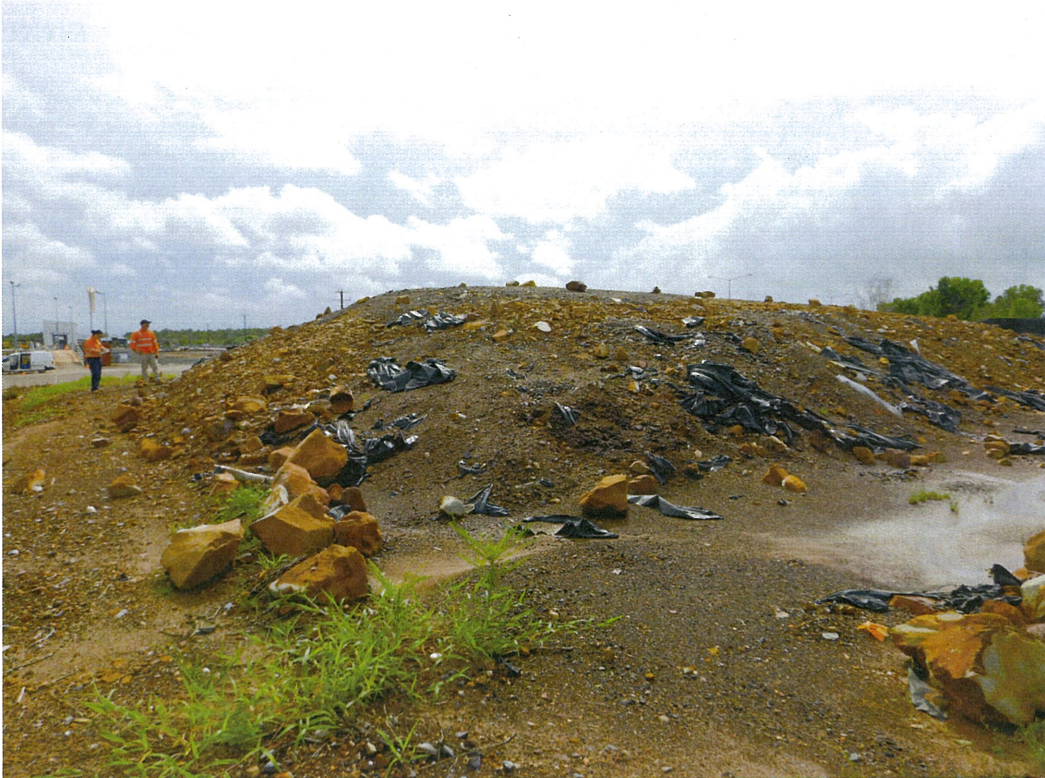
Photograph 1: Stockpiled material facing east. Stockpile is uncovered with no erosion or sediment controls in place.
