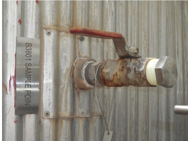
Figure 9-3: Example of Air Emission Sample port
