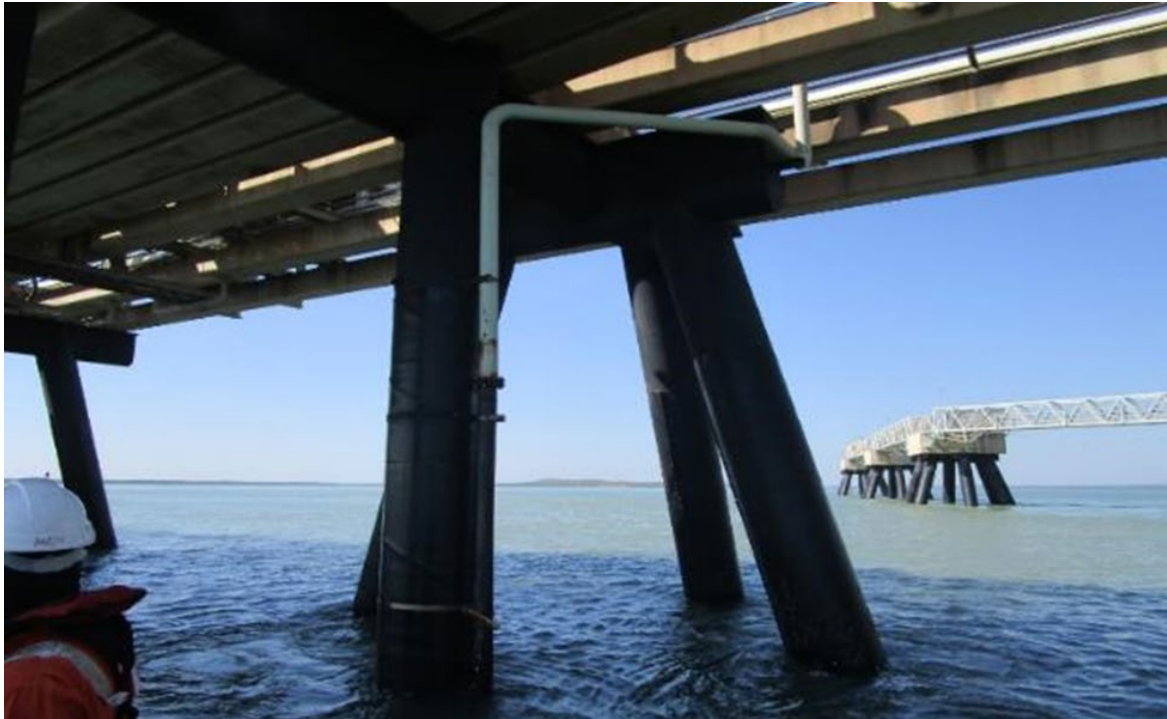
Figure 3-2: DLNG jetty outfall pipe (secured to pylon)
