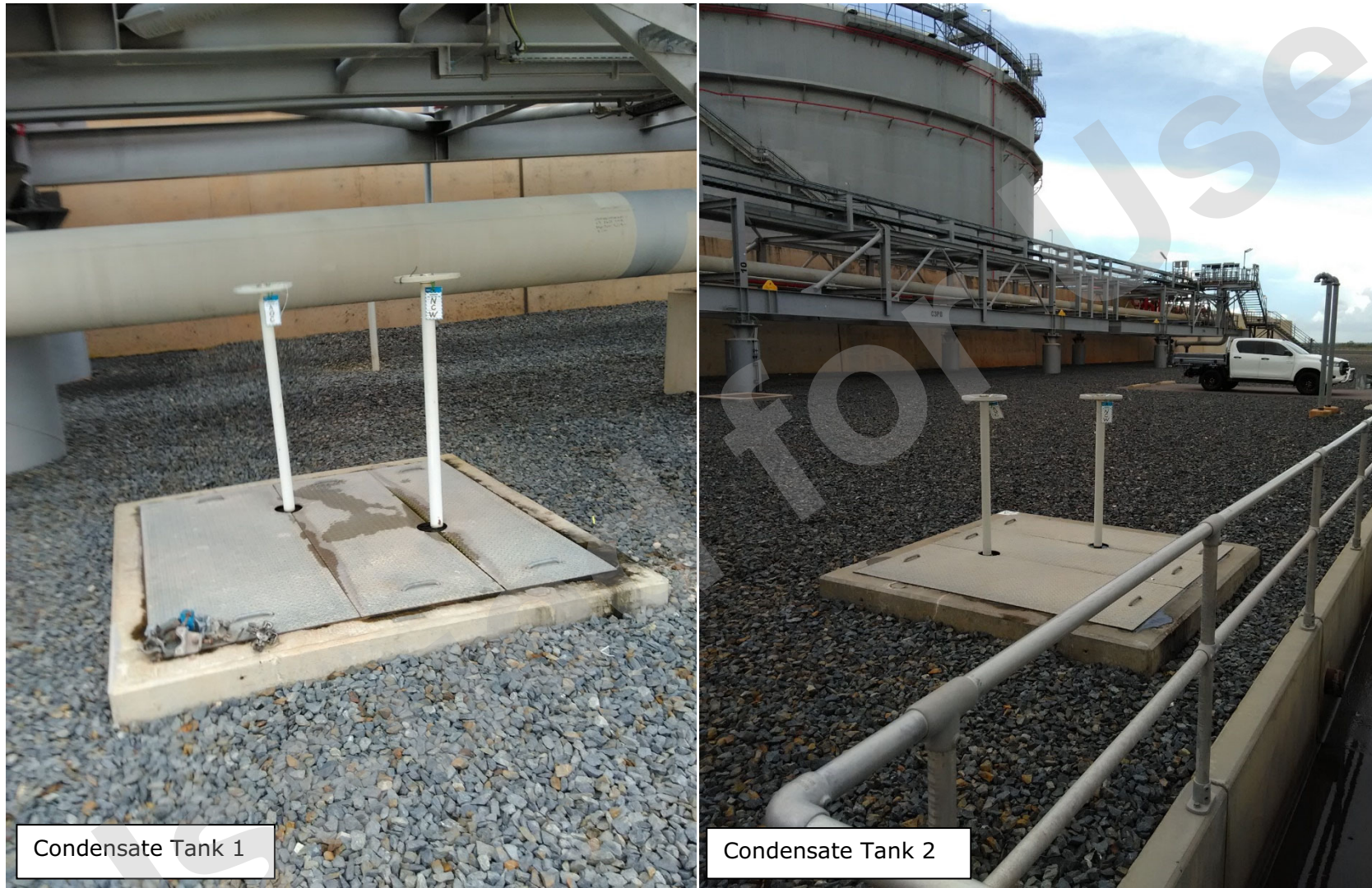
Figure 4-1: Condensate tanks bund drain isolation valves
