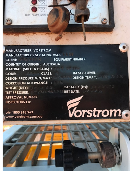
Figure 2-4. Volstorm tank compliance plate
