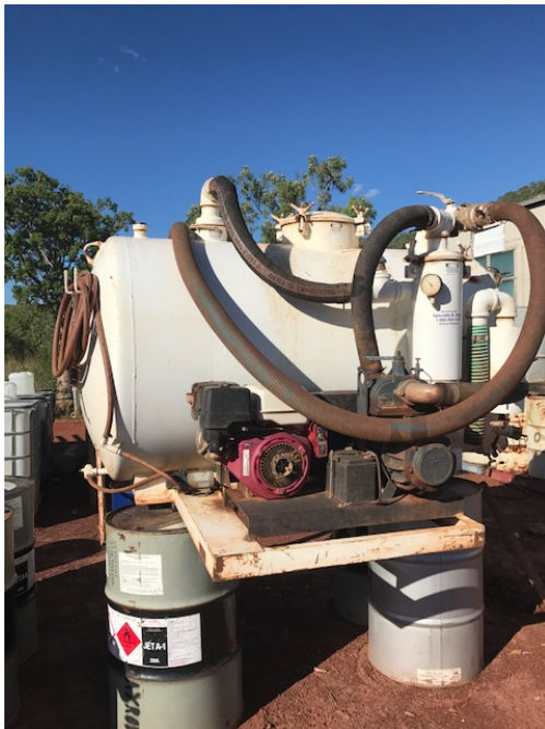
Figure 2-5. Jurop 2,000 L tank
