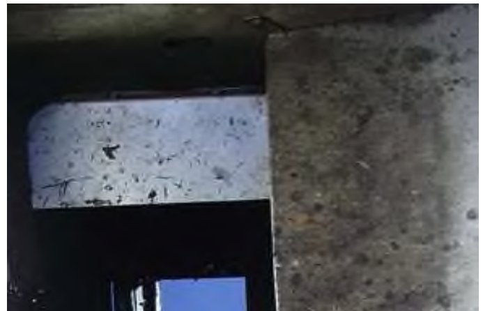
A view of the unit after being cleaned
