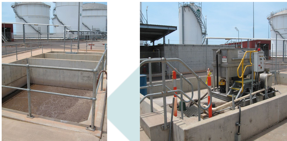
Figure 3: Baffled sediment and oil trap (left) and Oil Water Separation System (right)
